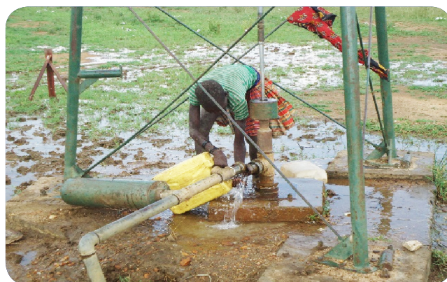
Leaking pipes at the partially restored windmill for pumping water in Lokitalebeu sub-county, Kotido district
