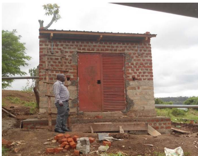
A water pump house constructed at Njeru Stock Farm in Buikwe District
