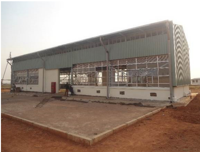
Construction of mechanical workshop at the Cotton Dressing Station in Pajule Sub-county Pader District at 80% completion
