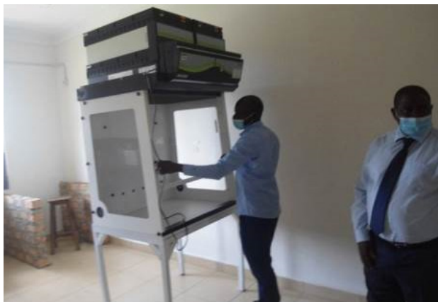
Installed fume hood purchased by UCDA with weak legs and a structure is being put up to be as base at NaCORRI
