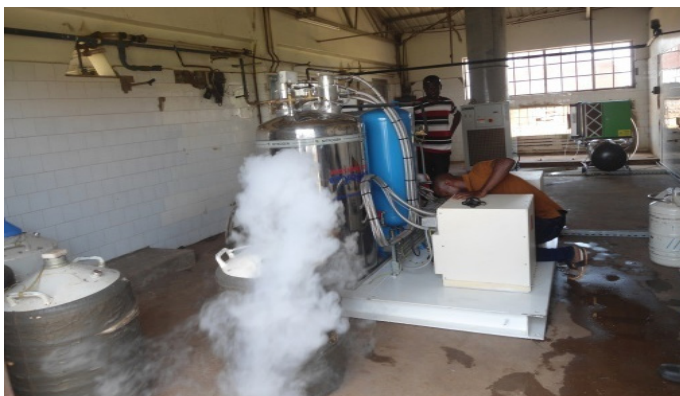
Nitrogen plant installed and in operation at Kiryowa Village, Njeru Municipal Council
