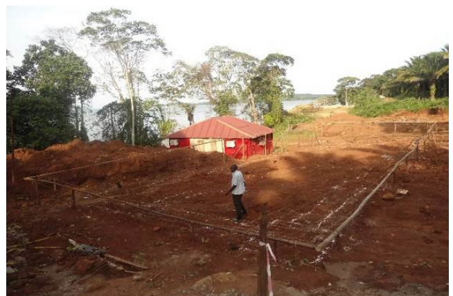
Works at Bugala Ferry Landing site in Nkusi Village had stalled for more than two years and were at 8% completion
