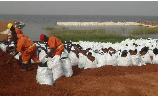
Kofa dam being established at Kiyindi landing site in Buikwe District to hold back water from the building site
