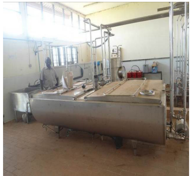
Milk cooling tank installed at the DDA Entebbe Dairy Training School in Entebbe Municipality Wakiso District
