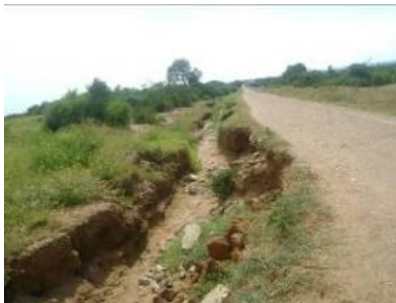
Heavily eroded side drain along Bukumi – Butyaba road
