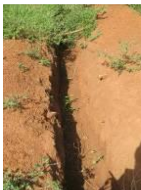
Trenching done but left uncovered posing a health and safety risk, Madi Opei RGC, Lamwo district
