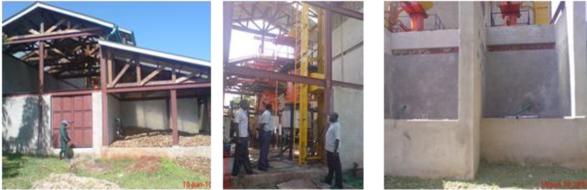
Nyabyeya Forestry College: incomplete walls and wood storage areas (left); building not wide enough for the machines (middle); concrete works in water cooling area are not waterproof (right)
