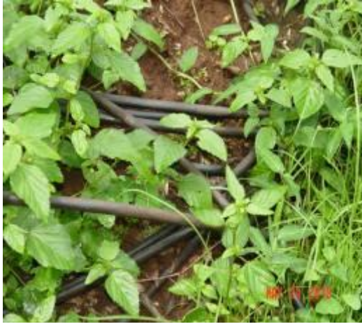
NBI Cables at the Tororo Site
