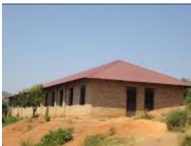
The 3 classroom block with a hall and store that was roofed with funding from the Presidential Pledge.
