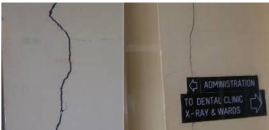
Cracks in the administration building
