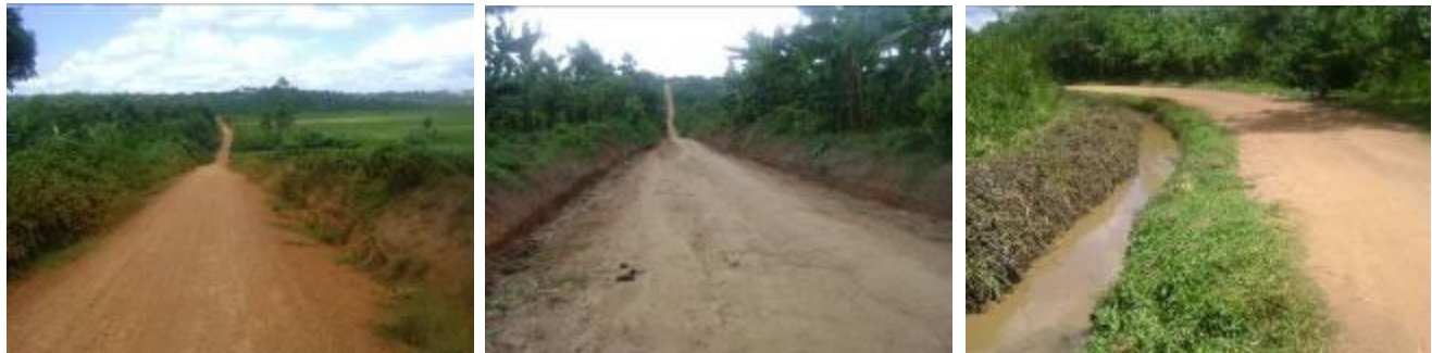
A completed section of Buswabulongo – Nama road, still in good condition (left); a bush cleared section of Nsozibiye – Kiwawu road under LGMSD (center); and a section of Wabiyinja – Nsozibiye road with a manually opened side drain (left).
