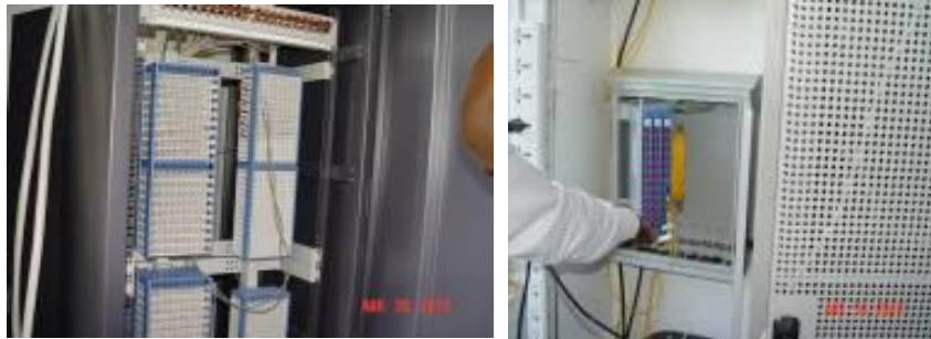
Equipment installed at the Foreign Affairs ministry
