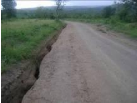
Graded section of Endiizi – Nyabyondo road with an eroded side drain
