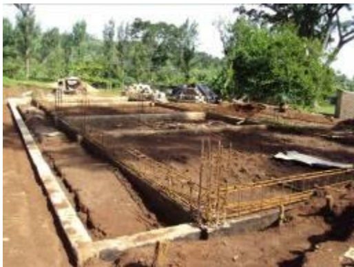
A storied classroom block that had stalled at plinth level at Masaba S.S.
