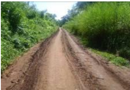
A section of Kasala – Kikunyu road with overgrown shoulders and slippery surface
