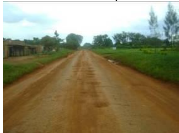
A section of Masindi – Biso road with potholes
