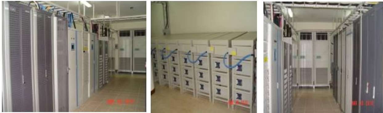
Servers, switches and battery bank installed at NITA-U secondary data centre
