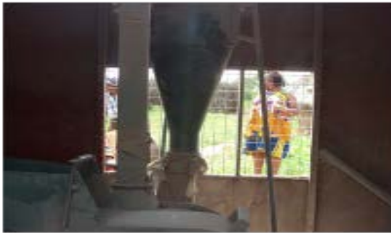
Installed and functional grinding mill in Ngoloriet sub-county, Napak District
