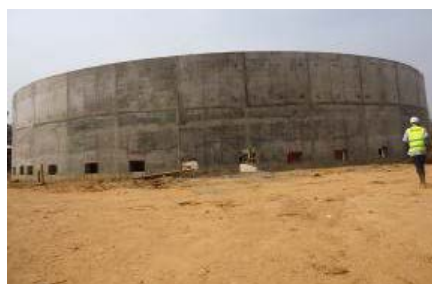
A Trickling filter at Bugolobi, Kampala
