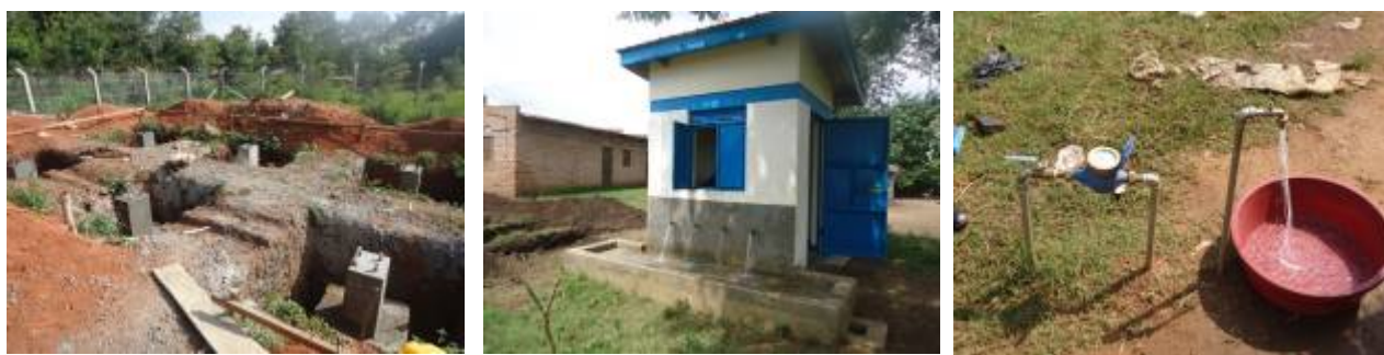
L-R: Stud columns for reservoir tank of Amach WSS in Lira district; Functional water kiosk for Dokolo WSS in Dokolo district; Functional private yard tap of Amolatar WSS in Amolatar district
