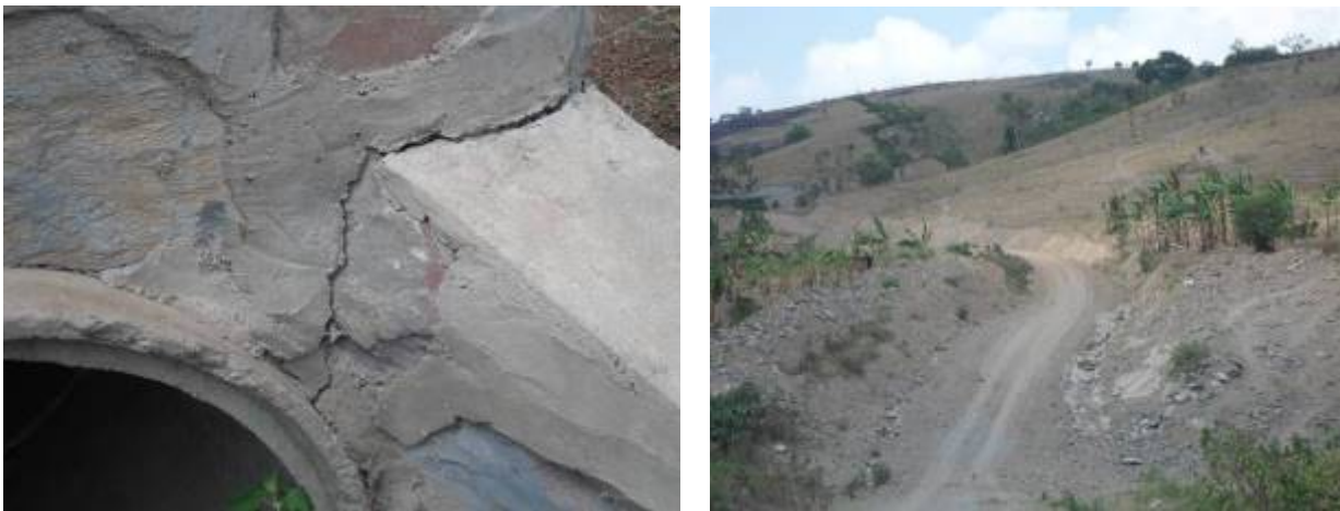
Cracked culvert along the Dyangu – Kitaliza – Kayanja road section
