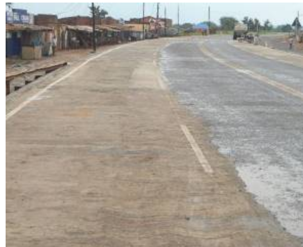
Atiak–Bibia road: Completed road section with concrete shoulders at Km 91+400 in Bibia Town
