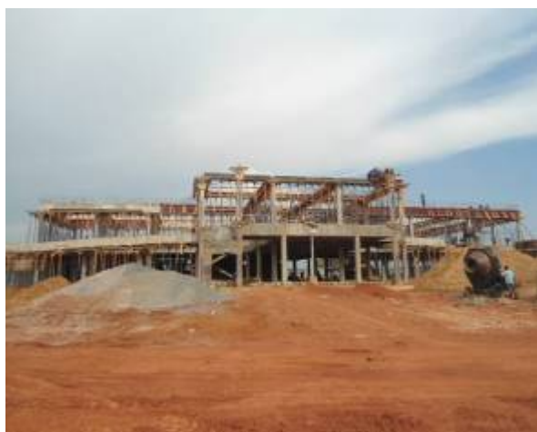
Construction of the main administration building at Elegu One Stop Border Post
