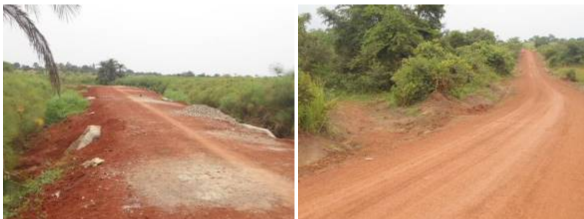
Left: A raised swamp section at Km 4+100 along Koro-Rom-Pece road; Right: A gravelled section with an off shoot drain along Palenga-Willacic (18km) road which was due for hand over
