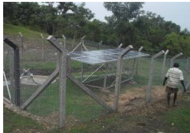
A completed solar powered irrigation system in Okuko sub county Arua district
