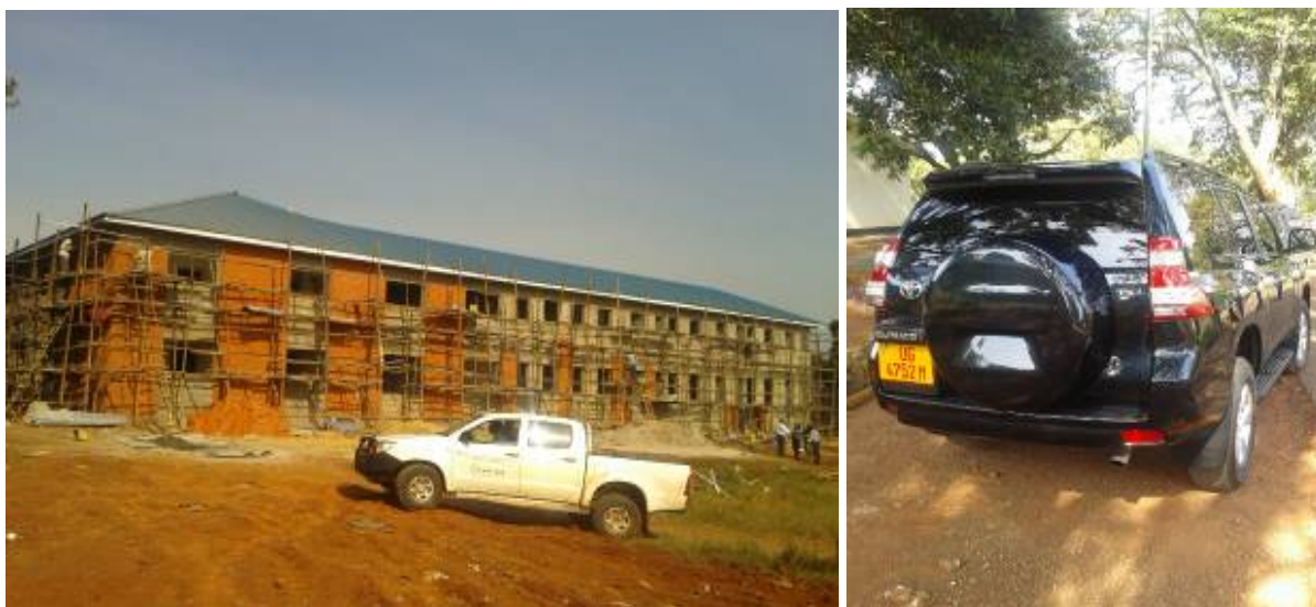
Left: Expansion works of the private ward at Butabika Hospital. Right: Newly procured station wagon at Butabika Hospital
