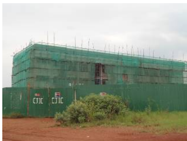
Construction of the administration block at UPIK that stalled
