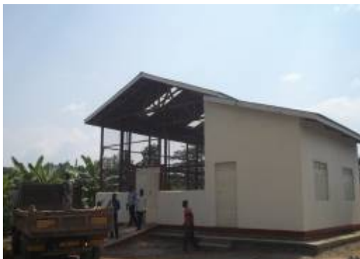
Ongoing construction of an abattoir at Nagongera Town Council in Tororo district by 13th August 2016
