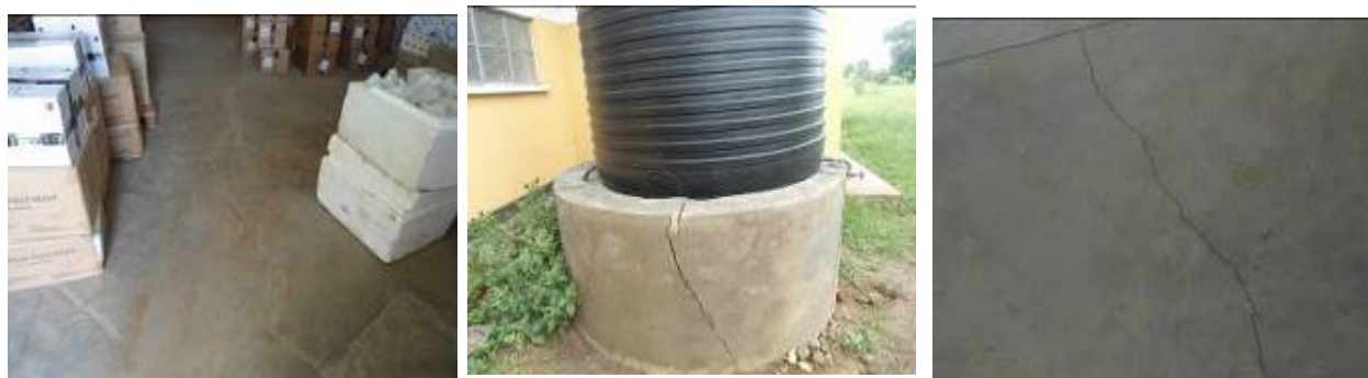
Left: A cracked floor at Nebbi DHO store; Middle: Failing tank stand at Kumi HCIV; Right: A cracked floor in a general ward in Mpongi HCIII in Pallisa district
