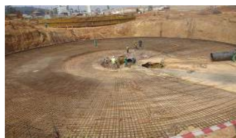
Base steel works for one of the secondary sedimentation tanks in Bugolobi, Kampala
