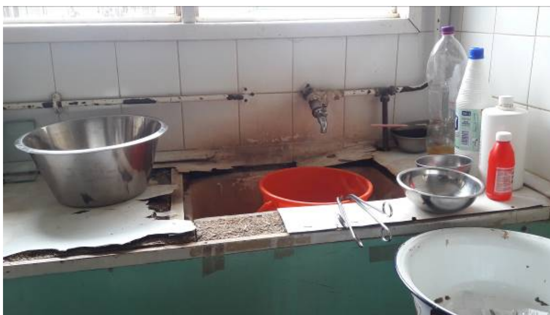
A sink at Pallisa General Hospital
