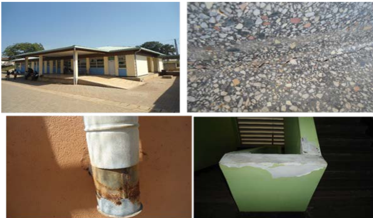
Left: Causality infrastructure at the Three million dollar project at Nebbi Hospital Right: Cracks in the floor, rusting Chimney at the attendants kitchen and paint peeling paint in some of the T-block at the same hospital
