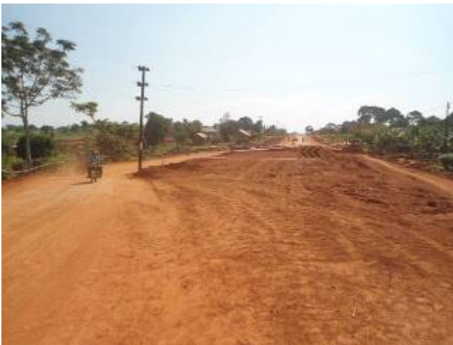
REA electricity poles in the middle of the project road at Km 21+600 on Misuta–Lumino road
