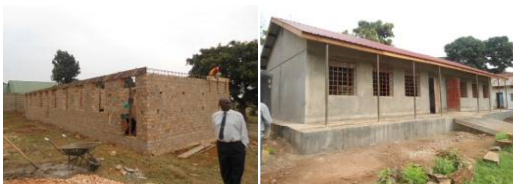
Left: A classroom block at Gayaza CoU at ring beam, Right: A classroom block at Mityebiri SDA at finishes level
