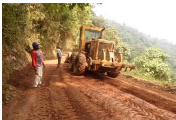
Gravel being spread along Ikumba – Nfasha road maintained under term maintenance contract
