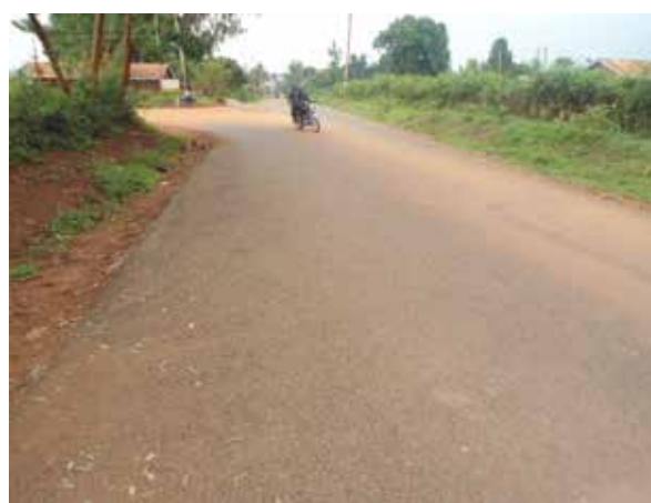
A section of the newly surfaced Malukhu Road with Jet Patch technology for sealing works
