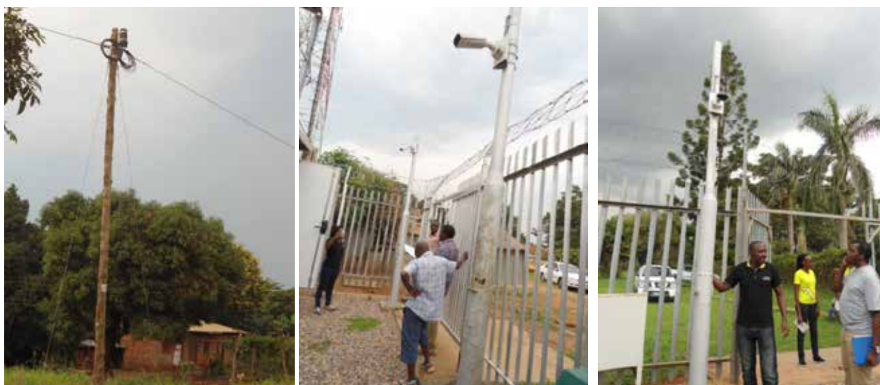
L-R: OFC strung along Hoima-Kyenjojo route and installed CCTV cameras at Masaka and Masindi Transmission Sites of the NBI
