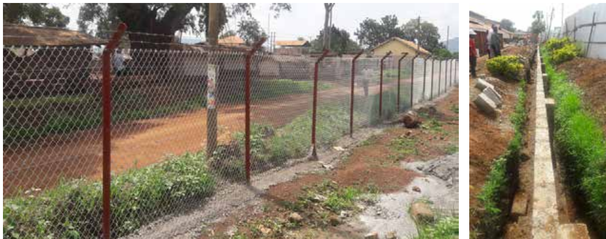
L-R: Chain link at Fence; Block wall under construction at Hoima RRH
