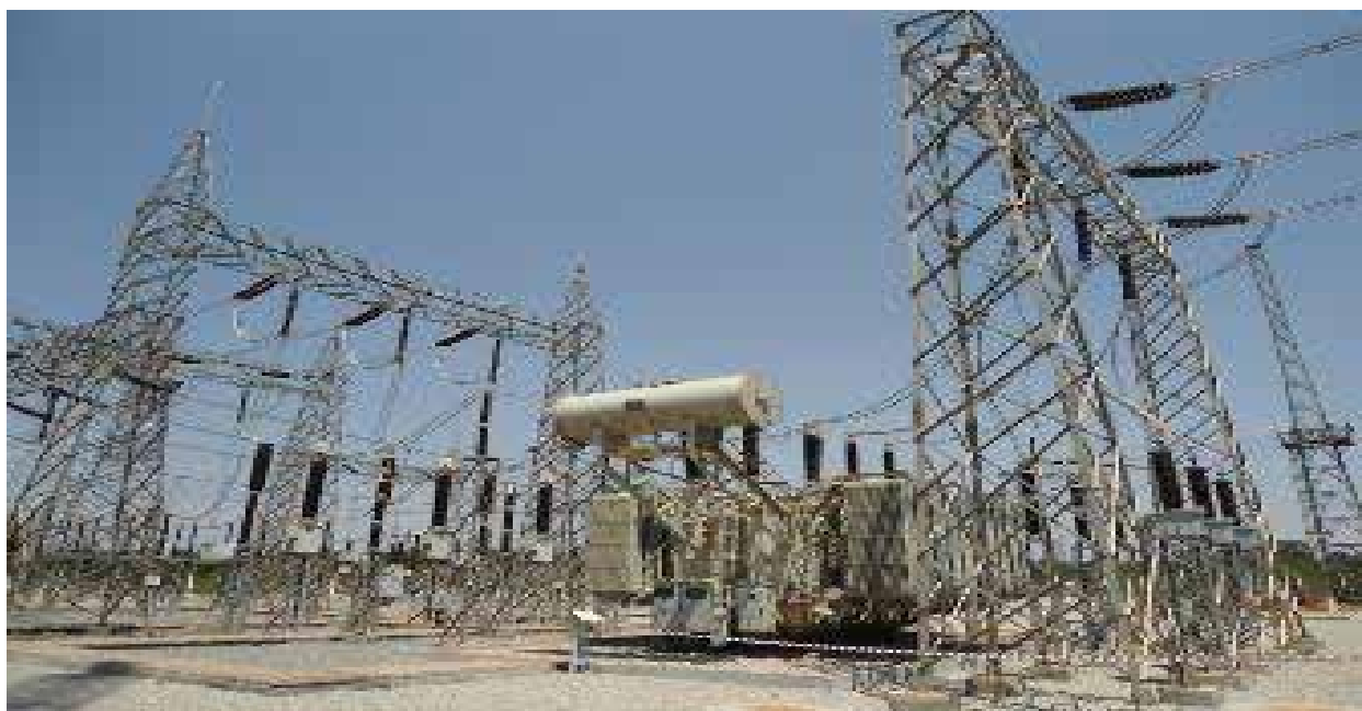
Fig. 1: Completed 132/220kV switch yard at Bujagali substation
