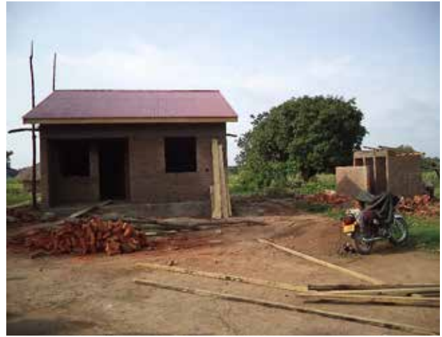
Ongoing civil works on Mr. Ayok’s low cost two bed-roomed house, with a toilet and kitchen in Alebtong District
