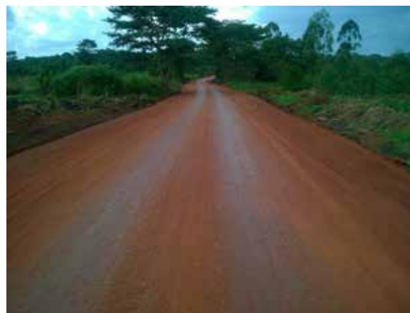
A well gravelled Kasiso–Mazzi–Kalungi Road implemented under periodic maintenance contract – Luweero station
