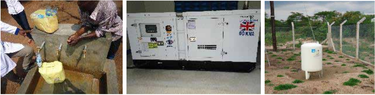
L-R: A public stand post at Kakooge WSS in Luwero Town Council, Luwero District; Generator at Mijeera WSS in Mijeera Town Council, Nakasongola District
