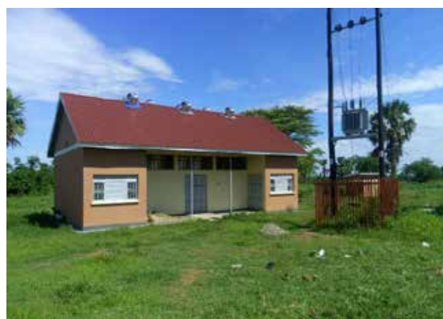
Installed power grid on maize mill facility at Ayer sub-county, Kole District
