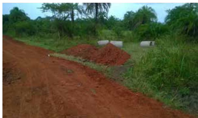
Culverts yet to be installed at the swampy Section of Namusaale – Lusanja Road
