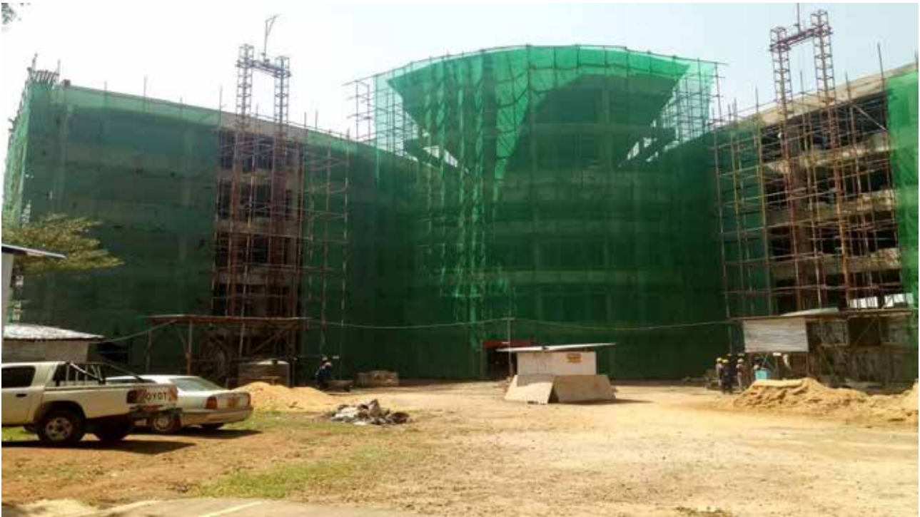
Ongoing works on the new offices for the Petroleum Directorate in Entebbe
