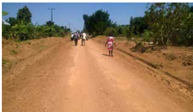
A well graded section along Kyesiga-Malembo Road implemented using Force Account – Masaka station
