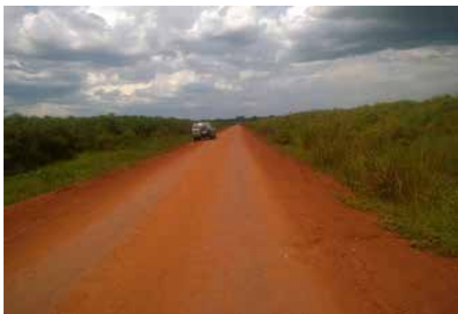
A well graded Ziobwe - Kabimbiri Road implemented using Force Account – Luweero station
