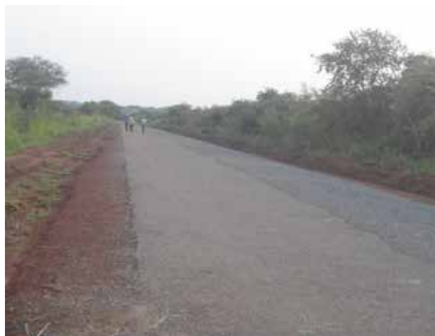
A sealed section of Lyandyang Road
