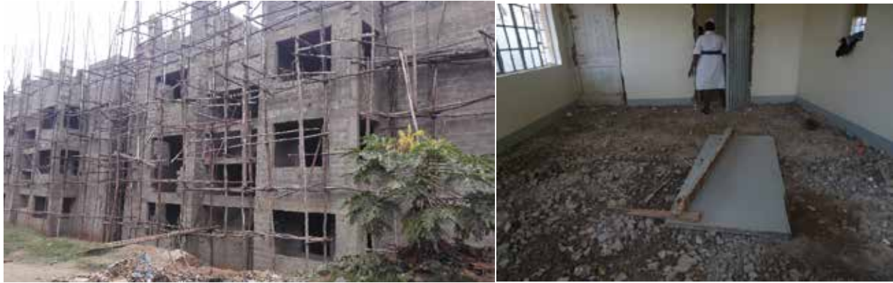
L-R: Staff houses under construction; Screeded floor in refurbished laboratory and orthopaedic offices at Mbarara RRH
