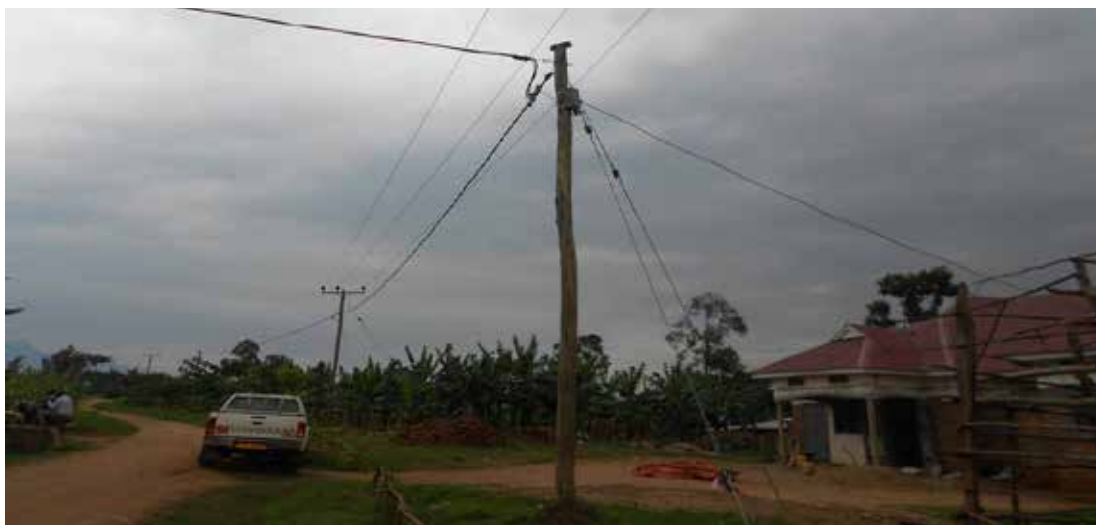
A homestead, newly connected to the completed GoU funded electrification scheme in Sironko District
