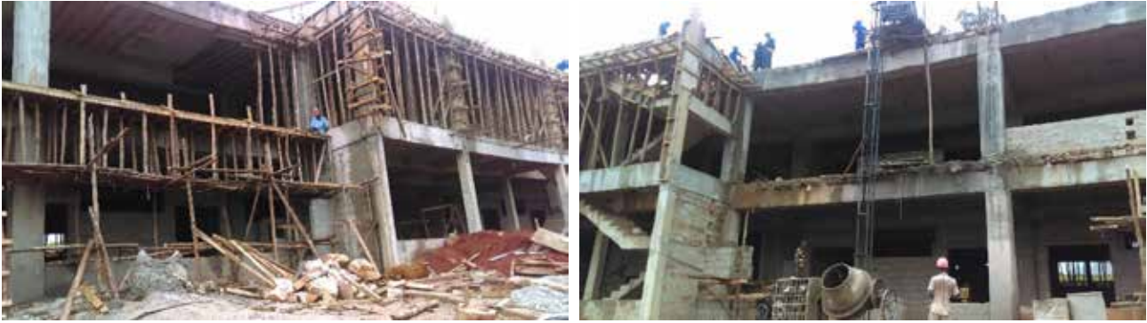
Ongoing construction works of the Central Lecture Block at 45%, progressing on schedule
