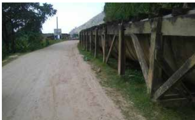
Completed section along the Nkenda Bugoye Nyakalingijo Road implemented using a periodic maintenance contract- Kasese station
