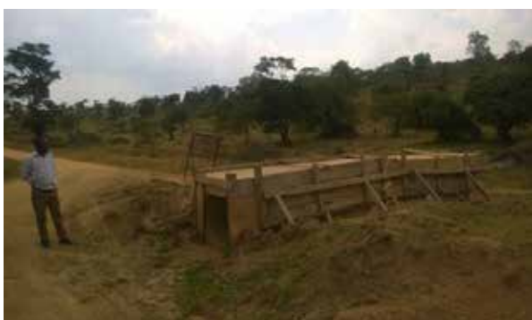
An incomplete cross culvert along Kasambya – Nabakazi Road requiring gravel for backfill – Mubende station
