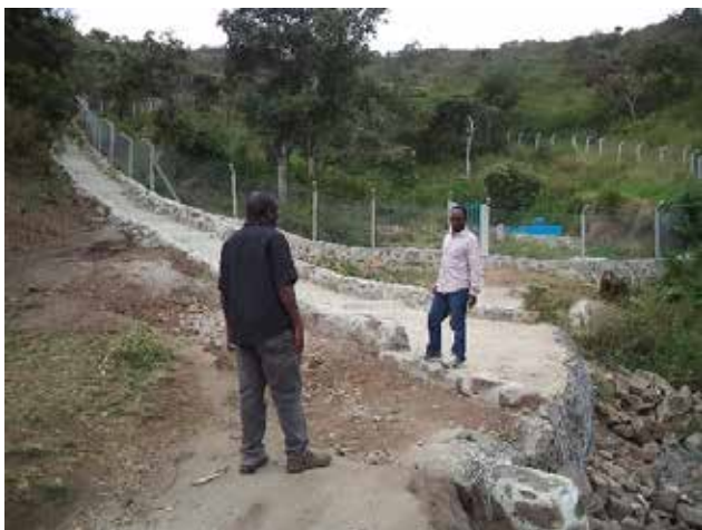
Murema water scheme in Kashumba sub-county, Isingiro District
