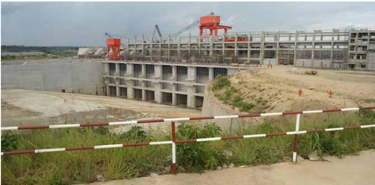
Ongoing works at the tail race end of Isimba HPP showing newly installed overhead crane gantries
