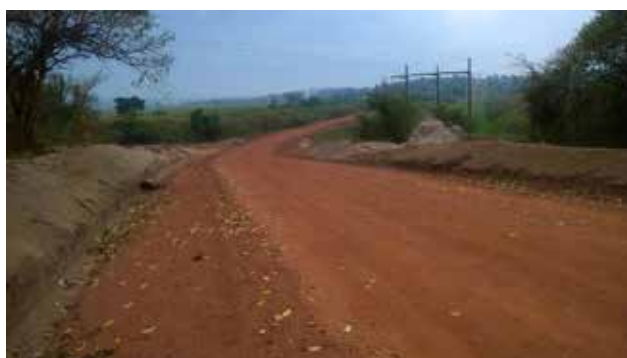
A well graveled section of Lusalira-Nkonge Road implemented under term maintenance contract – Mubende station
