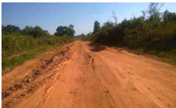
Deteriorated section along the Kyapa – Kasensero Road due to abandonment of works by the contractor for over 10 months
