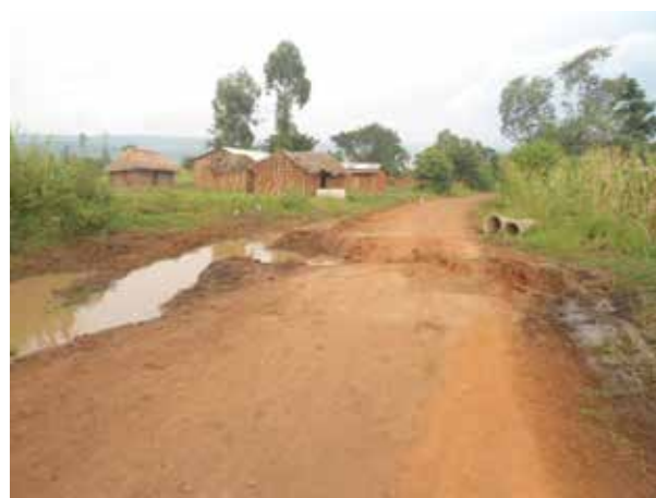
A broken culvert at km 0+500 along Buyaga-Muyembe Road
