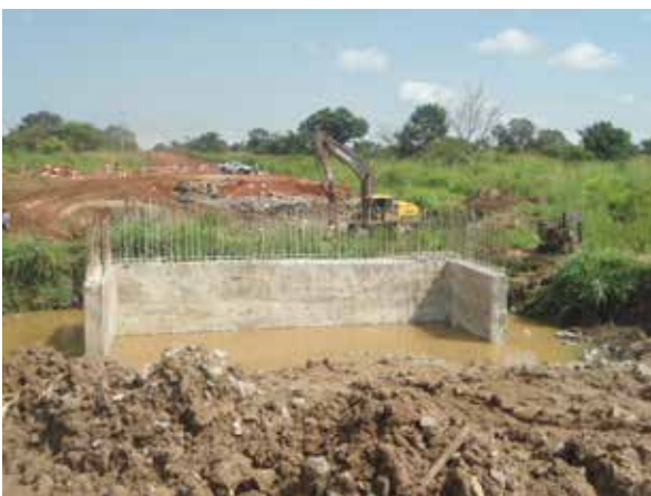
Construction of one of the bridge abutments at Km 25 along Olwiyo-Gulu road
