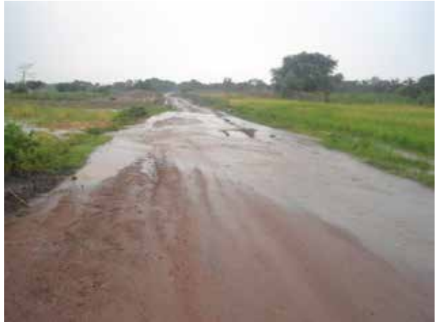
A section of Kalamira-Kagulu-Izimba Road affected by water
