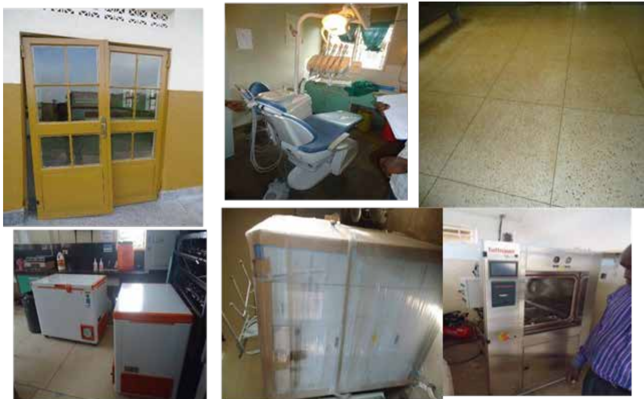
Clockwise: broken door Padibe HCIV maternity ward, Dental unit in Palisa hospital; Defective terrazzo Iganga GH OPD, Auto-clave Kitgum Hospital un-installed washing machine Apac GH and Installed solar
