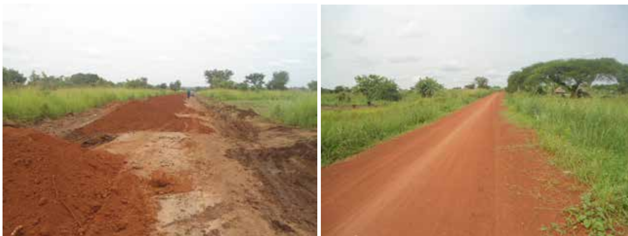
L-R: Dumping of gravel for the gravelling activity along Cwero-Omel-Minja road, 42km in Gulu district; A completed section of Minakulu-Okwir-Koroba road, 10.5km in Omoro section
