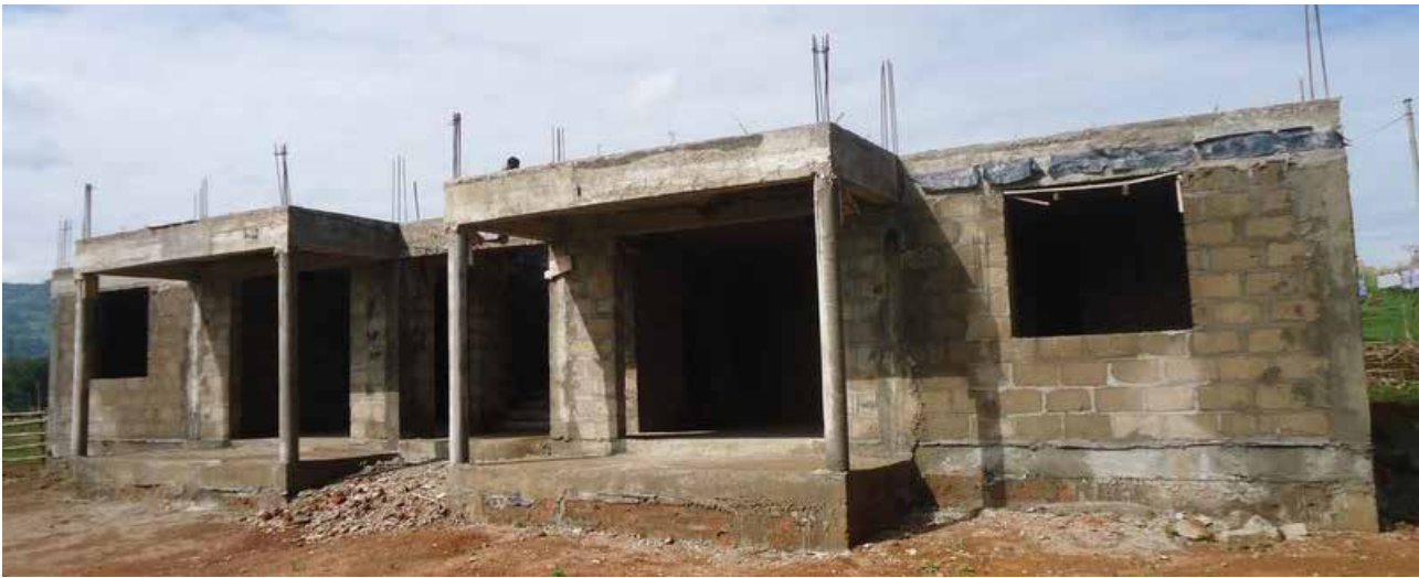
Stalled staff house at Kapchorwa Hospital
