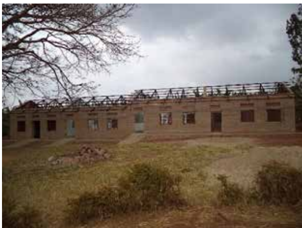
A three classroom block with staffroom at Rugaaga Primary school, Rugaaga sub-county
