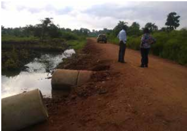
Incomplete culverts installed along Luwube-Grammer-Sekamuli Road
