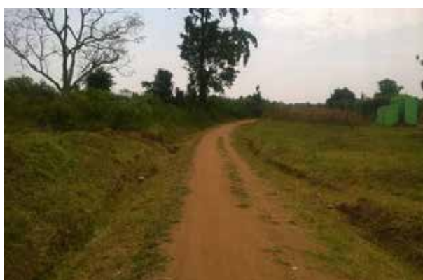
Completed section of Butoro – Sanga Road almost covered by grass- Mpigi District
