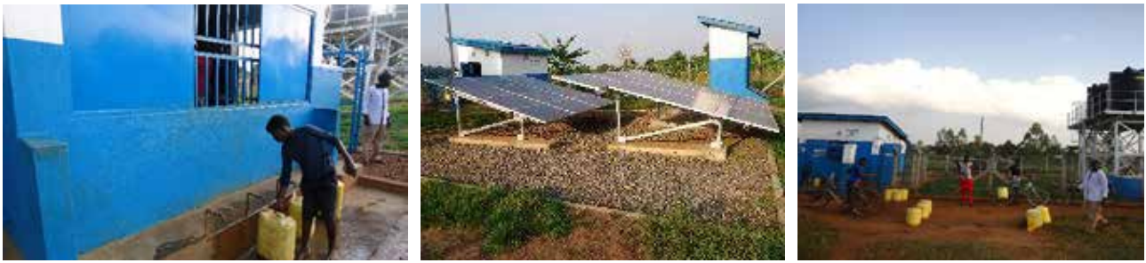
L-R: Public water kiosk; Solar array, Pump House and Ecosan toilet for Munduya Water Scheme in Daban sub county Busia District
