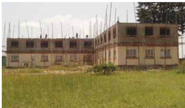
The Science block under construction at Kumi University as pledged by the President
