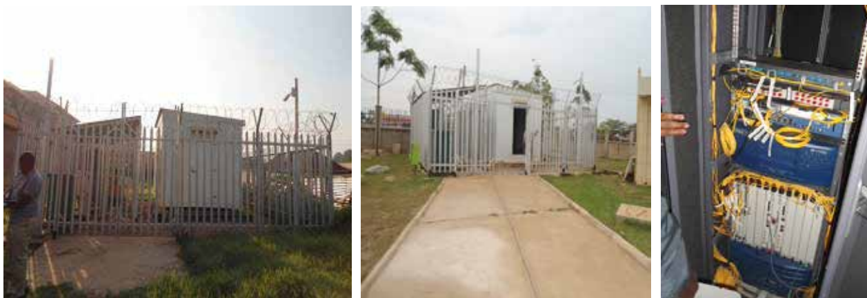
L-R: Completed NBI Transmission Sites (TS) in Kabale and Mutukula, and installed equipment at Mbarara TS all completed under Phase III of the NBI in 2017
