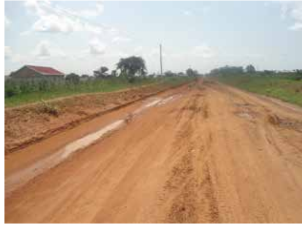
Deteriorated section at Km 3+700b along Arapai-Amuria Road
