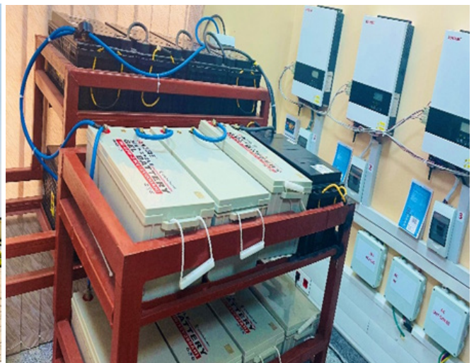
Power Backup system
