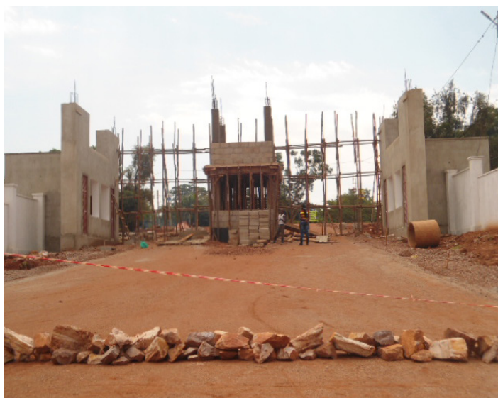
Works on the main gate at the West End at 50% progress at Kyambogo University
