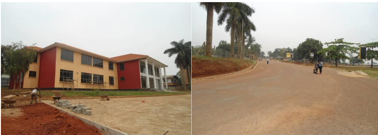
L-R: Construction of the Bursar's office; Part of the tarmacked 600 metres of the road at MUBS
