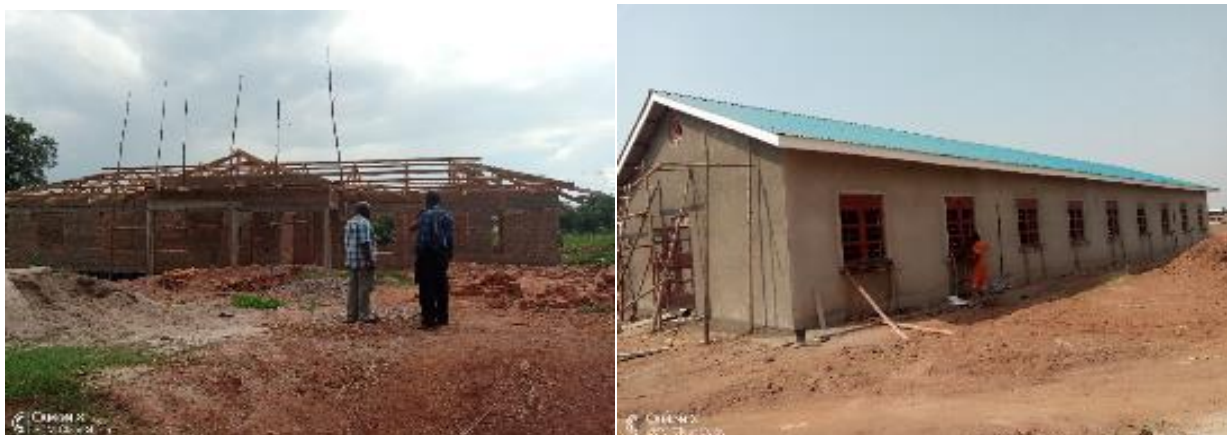
L-R: Construction of administration block at Jinja PTC in Jinja District at roofing stage; Construction of boys Dormitory at Kitgum Core PTC in Kitgum District at finishes level
