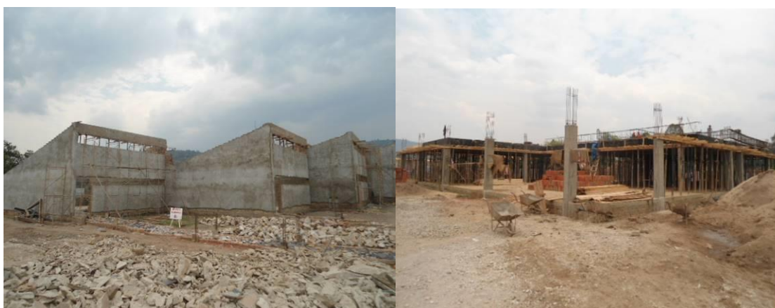
L-R: Renovation of the lecture room complex at roofing stage; Construction of the Library/Resource Centre at Kabale NTC as at January 2019
