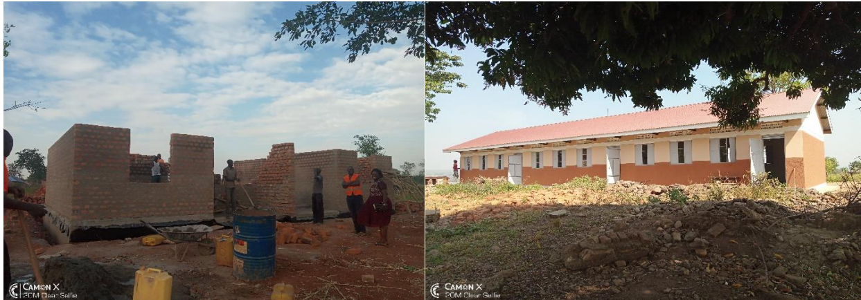
L-R: Construction of a two classroom block at wall plate level at Aringodyang PS, Iceme S/C, Oyam District; A 3- classroom block completed at Katrini P/S in Arua District
