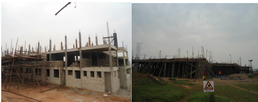
L-R: Construction of the students' hostel, and construction of the Faculty of Computing at Mbarara University of Science and Technology
