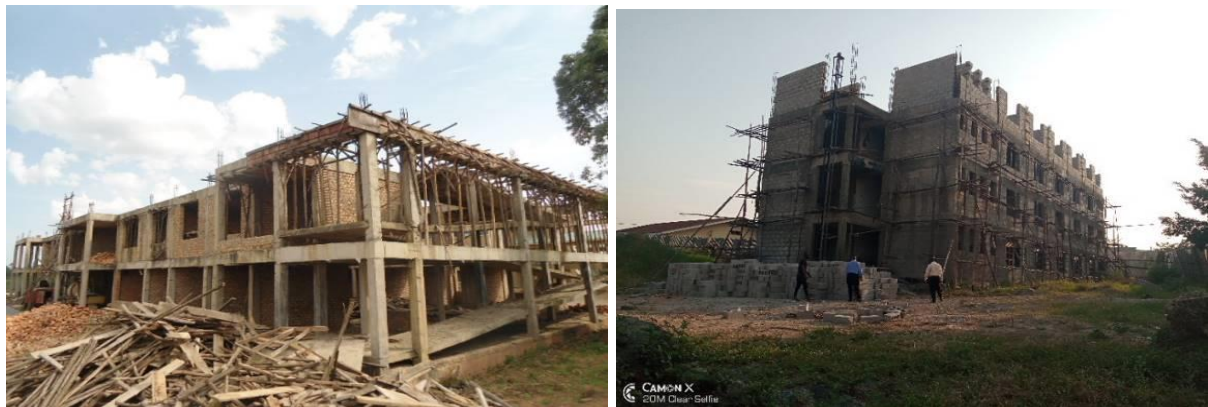
Left: Works on the administration block at UTC Bushenyi resumed after a 2 year stallment Right: Construction of a hostel block at Arua Comprehensive School of Nursing
