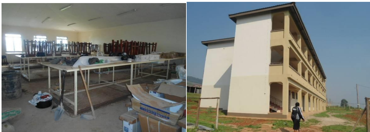
L-R: The biology laboratory under renovation: The General lecture block at Kabale University
