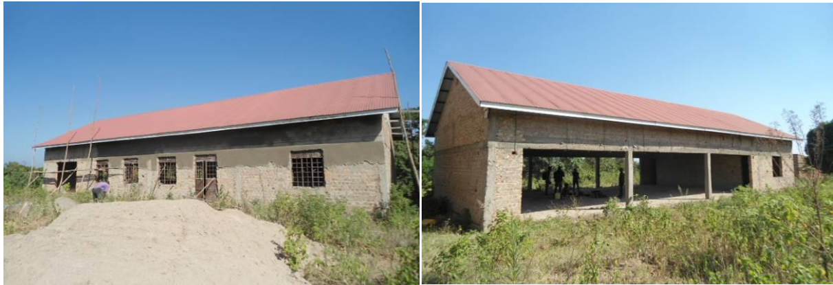
Civil works on all structures at Bamunanika Technical Institute resumed after 2 years' stallment. Plastering was ongoing on a 2 classroom block and a workshop block
