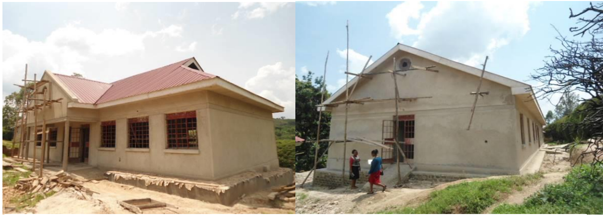
Left: Construction of an administration block at finishes level, Right: Construction of a dormitory at finishes level at Bikungu PTC, Mutara sub-county in Mitooma District
