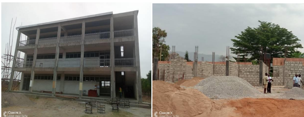
L-R: Lecture block at Arapai Campus in Soroti at final finishes; Lecture block at Mbale Campus, Busitema University
