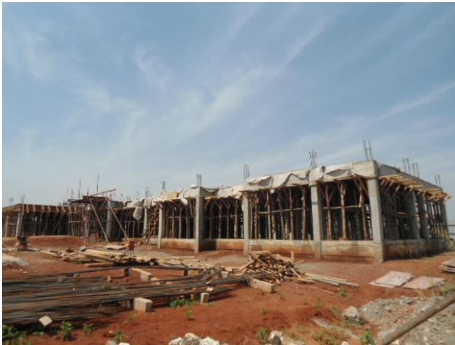
Civil works on the two storied male dormitory at 50% progress at UPIK
