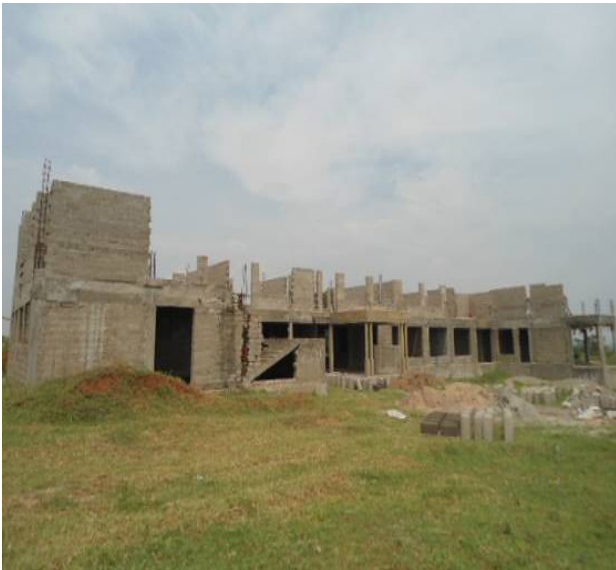
A 2 storied administration block that has been under construction since FY 2016/17 at 60% progress at UCC Tororo
