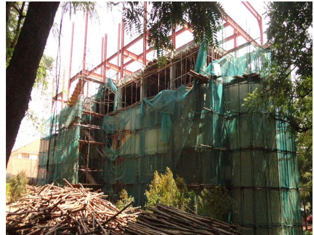
On-going extension of the Women and Gender Studies building planned to add three more floors
