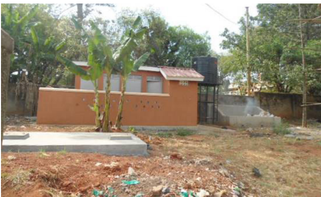
One of the 5 waterborne toilet constructed at Nkoma S.S in Mbale district
