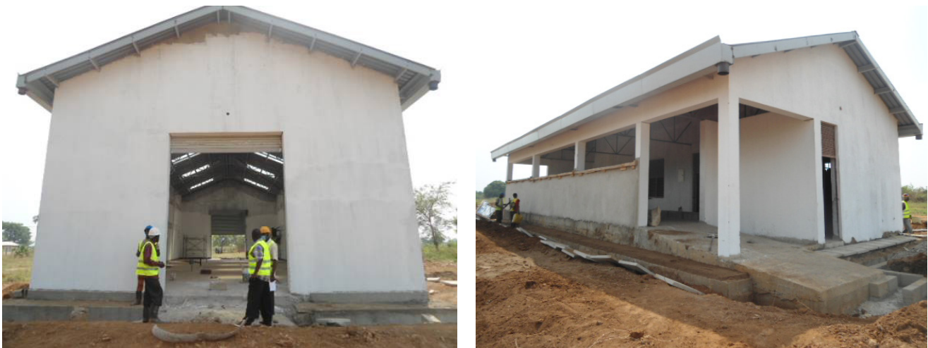
The Milk Process House at 79% and the Spray Race room at 78% progress at Kaberamaido TI
