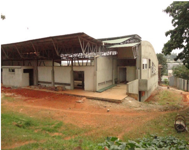
The indoor stadium being constructed by the Engineering Brigade of the UPDF
