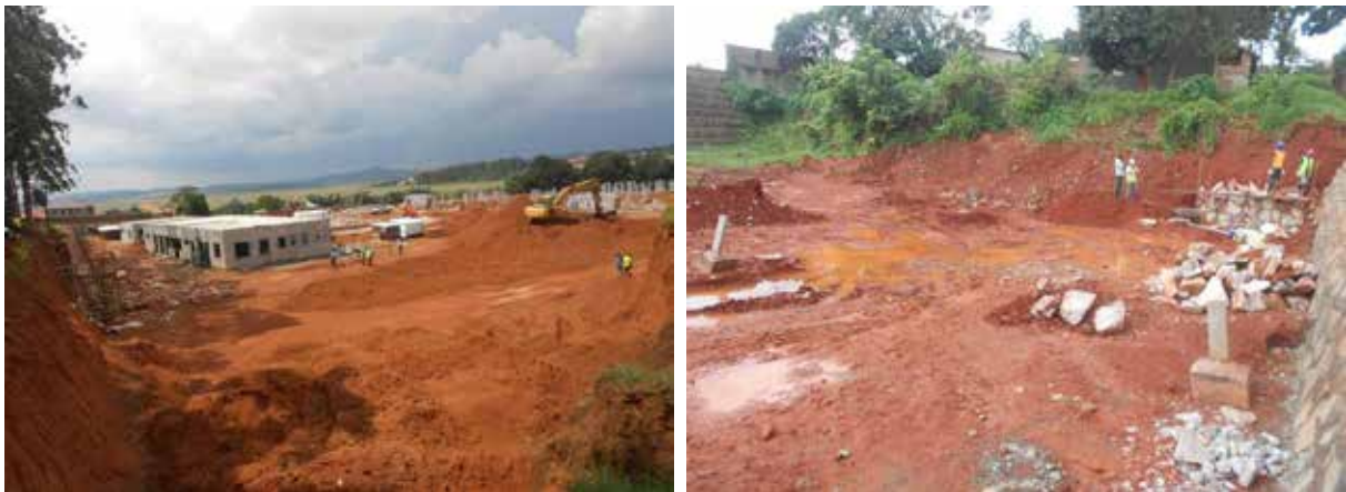
L-R: Civil works in progress at Entebbe substation; One of the completed tower foundations for the Mutundwe-Entebbe Line
