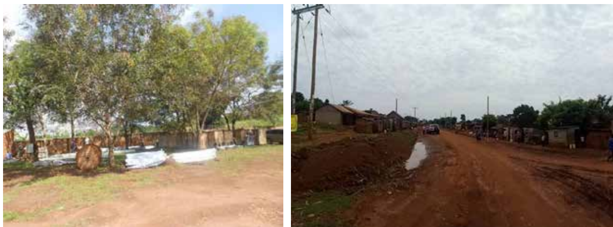
L-R: The contractors yard with the delivered materials at Namadope, Luuka; Ongoing stringing works at Bumana Trading Center, Luuka
