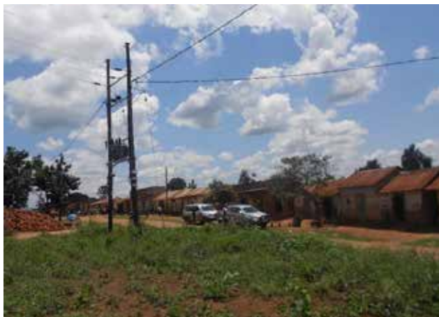
Left: A transformer installation at Rwobuhura, Kiruhura
