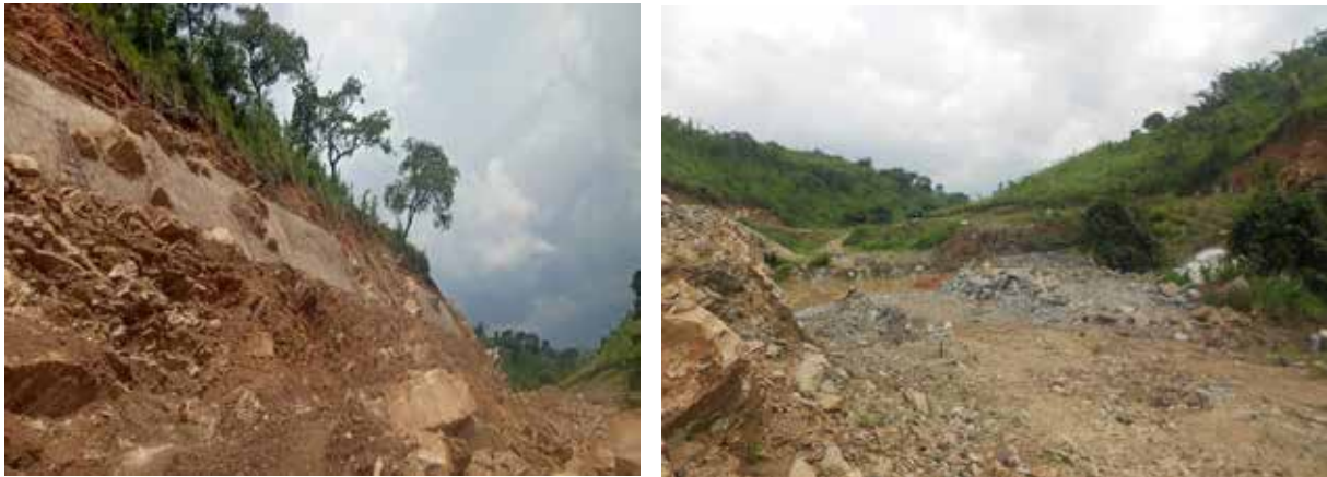
L-R: Slope protection works along the dam access road; Deep excavation at the dam site for Nyagak III HPP
