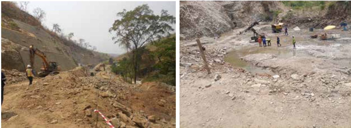
L-R: Slope protection works on dam access road; Completed excavated dam site
