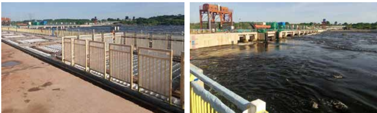
L-R: Installed guard rails at the Karuma HPP power intake; Raised water level at the Karuma Dam Intake
