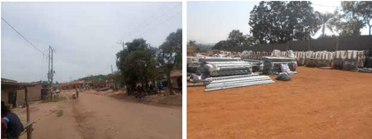
L-R: A completed scheme at Mbaare trading centre, Mbarara; Delivered materials at contractor's yard, Mbale
