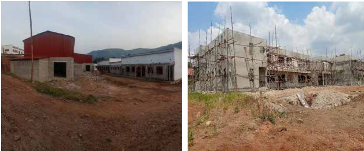
L-R: A view of works at the plant house and multipurpose halls at the Ntungamo Mineral Beneficiation Centre; Progress of construction works at Fort Portal Beneficiation Centre
