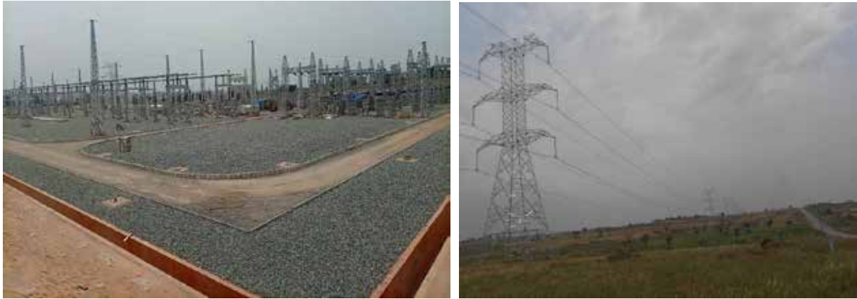
L-R: On-going elcteromechanical works a t the 400kV Olwiyo substation; Completed sections of the Olwiyo-Karuma T-line
