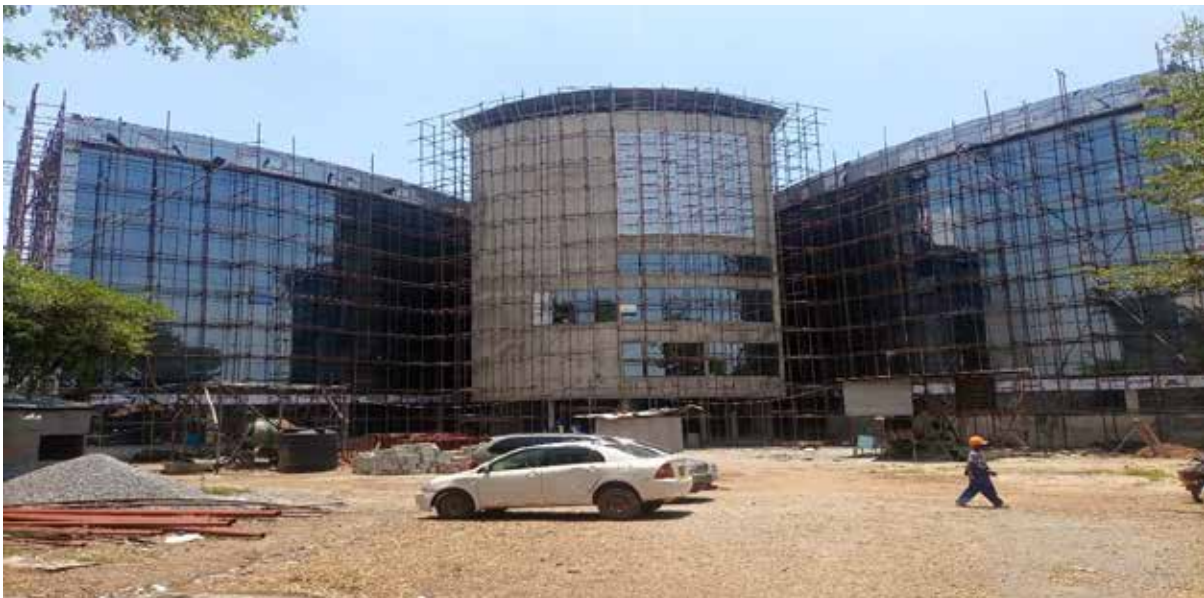
Phase three construction works for the new office building for the Petroleum Directorate and Petroleum Authority of Uganda (PAU)
