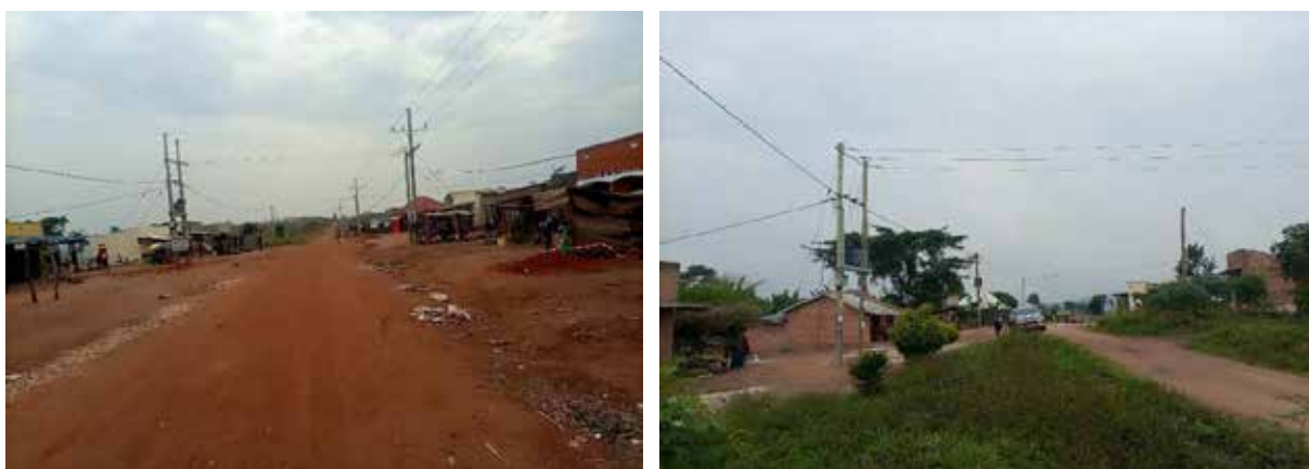
L-R: Advanced works under Kuwait Funding at Kamunana trading center, Kiryandongo; A completed scheme at Nadjoki Village, Nakaseke District under IDB III Lot 5
