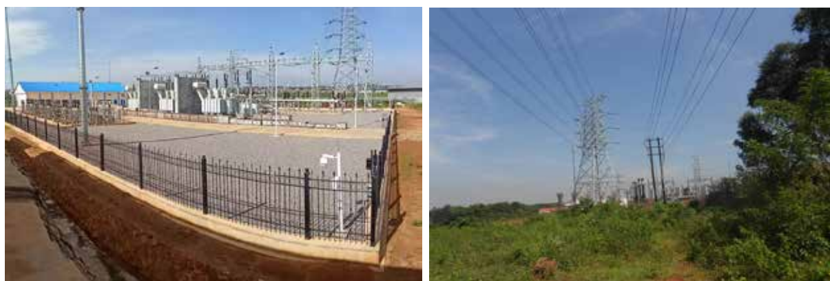
L-R: Completed and commissioned Namanve South substation; Completed Namanve South-Namanve North transmission line
