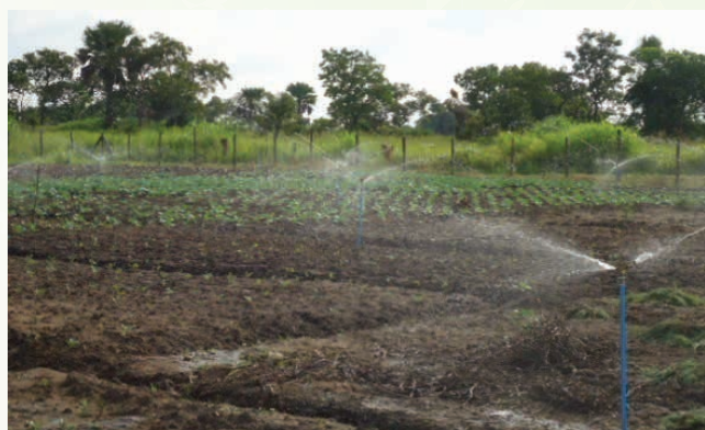
A sprinkler system of Ayweri small scale irrigation scheme in Gulu district
