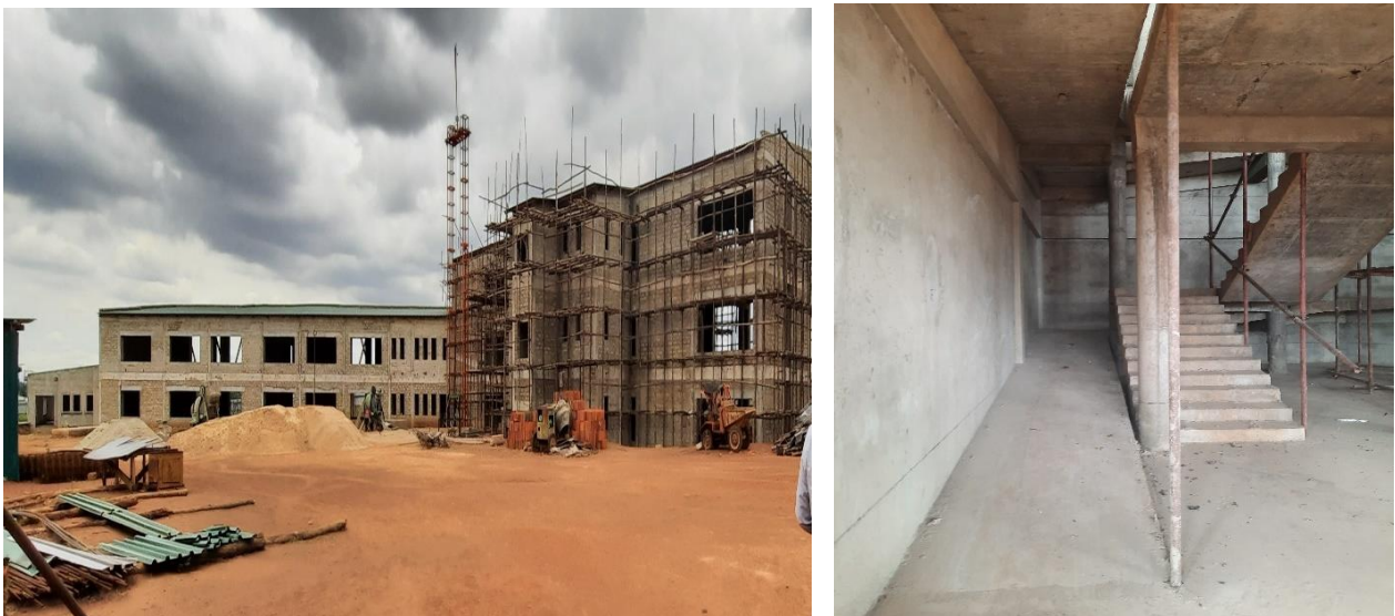
L-R: A rear view of the ongoing construction of the lecture hall, library and ICT blocks with overall progress at 73% and; a ramp provision for PWDs on the same block
