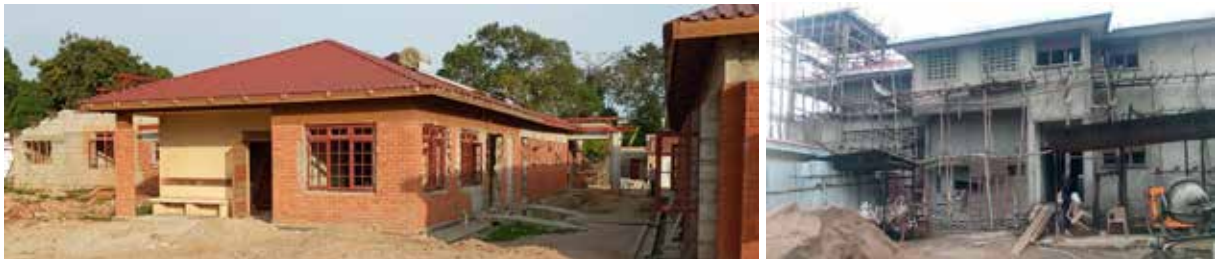
Left: Isolation Centre at Entebbe Hospital under renovation: Right: Status of works at Arua RRH EALPII Project
