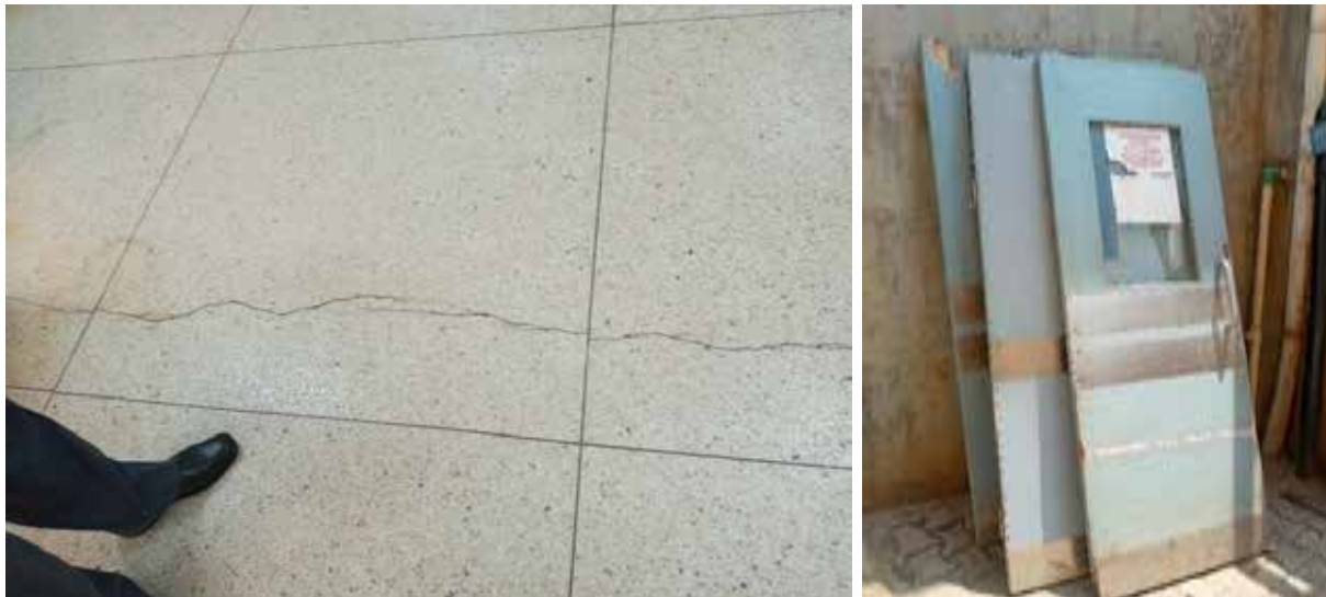
Left: Already cracked floor in the laundry room. Right: Some of the doors that fell off and not replaced at Kiruddu Regional Referral Hospital
