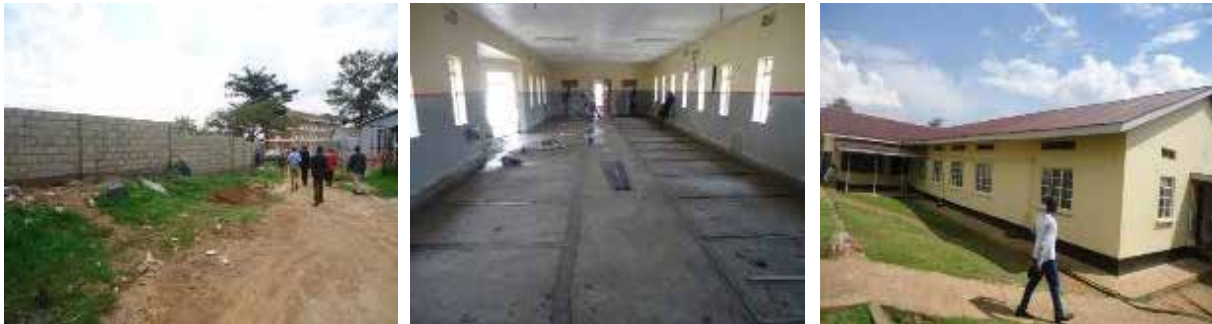
L-R: Perimeter wall under construction; Terrazzo works in the medical ward; and OPD substantially completed at Mbarara RRH
