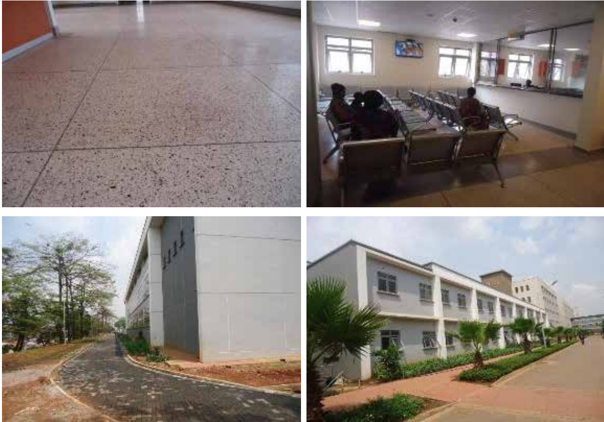
Clockwise: Failed terrazzo works, patients waiting for services at the private wing, Block D (private wing and paving works around Block K (new theatres)
