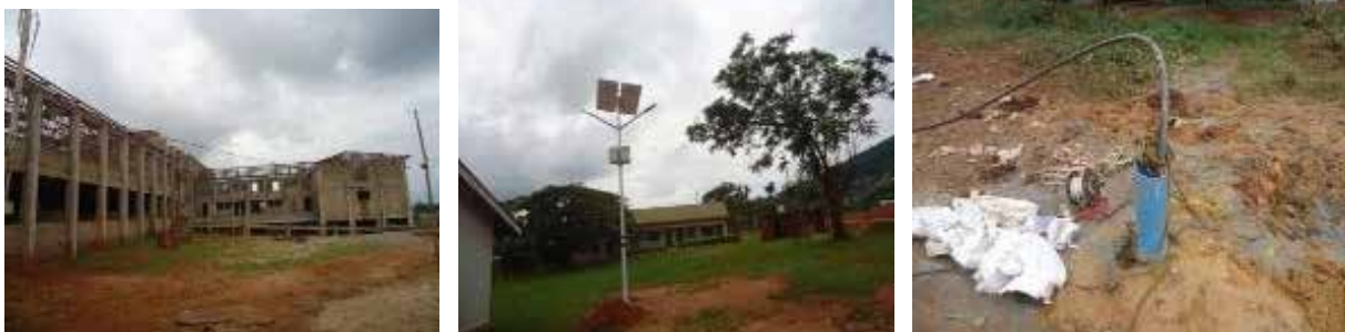
Pathology and paediatric complex under construction, solar security lights and submersible borehole procured and installed at Mubende RRH
