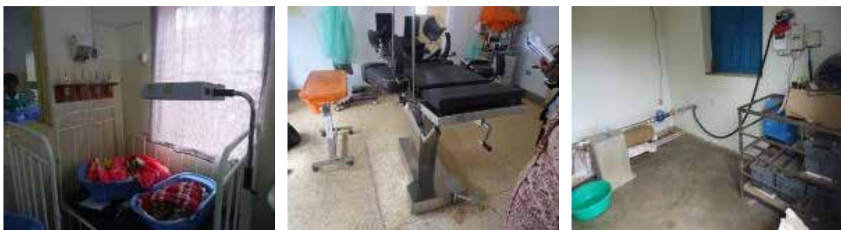
L-R: Piped oxygen in neonatal unit; operating table in the obstetric theatre; and water piping works at Hoima RRH
