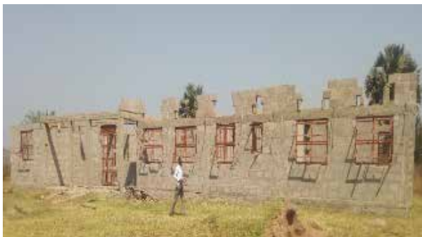
Rolled over project (FY 2018/19): Stalled maternity ward at Arinyapi HCII in Adjumani District
