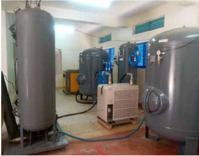
Oxygen equipment at Entebbe RRH
