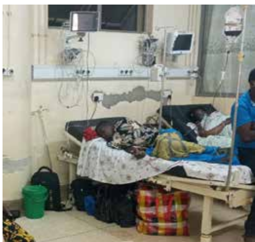
Oxygen service delivery points and conduits in the emergency ward of Kiruddu Hospital
