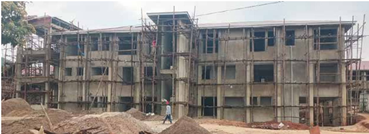
Front view of the Mubende RRH Surgical and Paediatric Complex under construction
