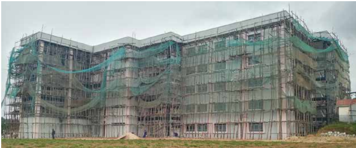
Front view of Maternity and Child Health Complex under construction at Masaka RRH
