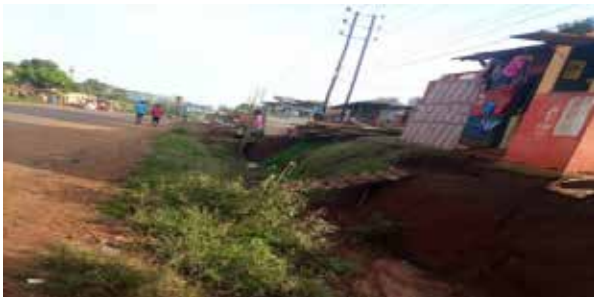
Kampala UNRA Station: A desilted drainage channel along at km 2+600 along Nazigo – Bukolooto Road however, the silt was returning fast and the channel was bushy
