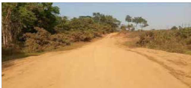
Hoima UNRA Station: A section of Kabwooya-Kituti Road at km 4+200 along Buseruka-Kigoroby Road
