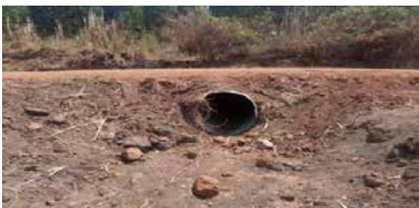
Hoima UNRA Station: An armco culvert installed at km 6+600 along the Buseruka-Kigoroby Road
