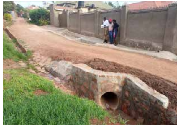
Mukono Municipality: A section of the road due for paving and a pipe culvert line installed on Kauga Road
