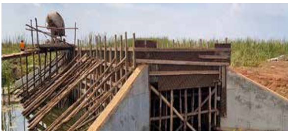
Jinja Station: Abandoned box culvert site at Lumbuye A -swamp crossing along Kaliro-Namwendwa-Kamuli Road
