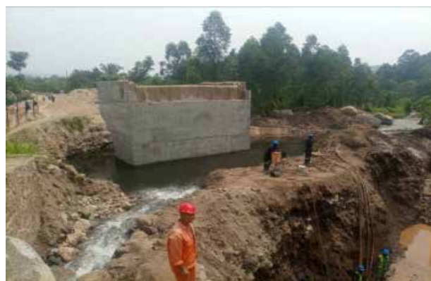
Excavation works for the second abutment on Kanyampara Bridge in Kasese District
