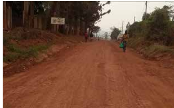
Hoima City: A section of Kiryabwire Road at km 2+200 where works were executed under routine mechanized maintenance
