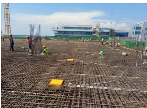
Entebbe International Airport: Ongoing slab works on the first floor of the New Passenger Terminal Building
