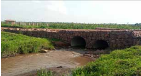
Kabale UNRA Station: Double Armco culverts installed along Rwentobo-Kisinga at the Uganda-Rwanda Border
