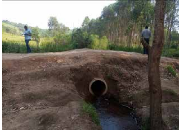
Mitooma District: An installed 600mm pipe culvert line with headwalls yet to be constructed
