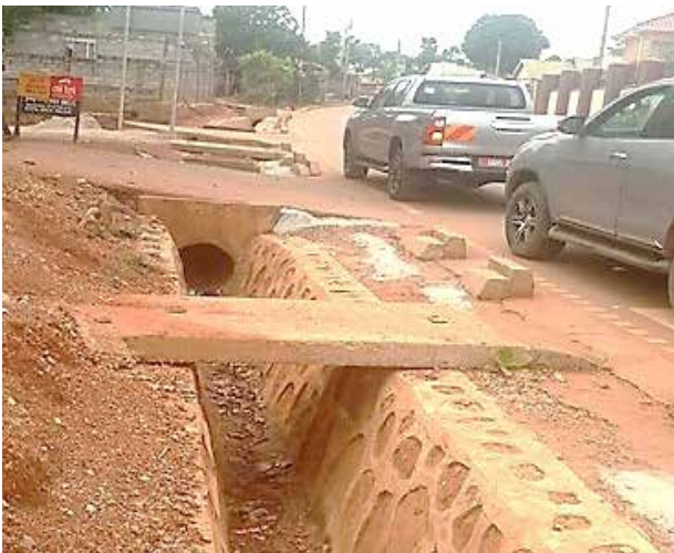
A completed section with access slabs of Entebbe Pediatric Hospital Access Road
