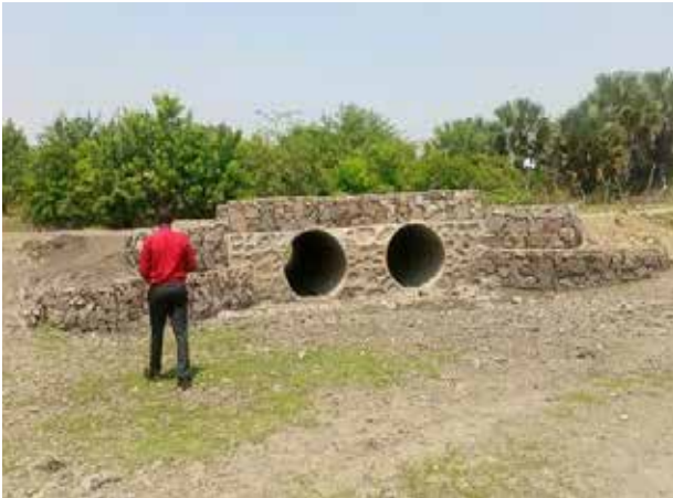
Ntoroko District: Twin Armco pipe culvert lines of 1.2m diameter (Kitogoto Bridge) on Butangama-Budiba Road. These were pending gravel fill
