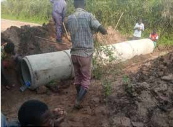
Gomba District: A section of Kawuula Maddu Road at km 4+600 with culvert installation works ongoing
