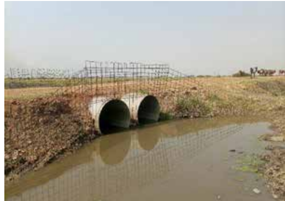
Ntoroko District: Pending headwall works on the double cell culvert at km 0+800 on Bweramule - Kayanja Road (4km)
