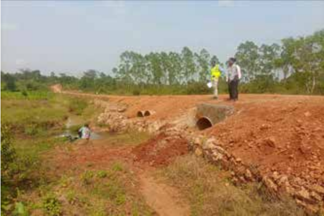
Wakiso District: Armcoculverts installed on Mawule - Nalusuga-Buwaga-Nabutiti-Kasozi Road (9.0km) in Nansana Municipality
