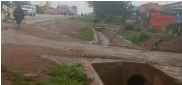
Masaka UNRA Station: A stone-pitched drainage section at km 21+500 along Masaka –Lyantonde paved road
