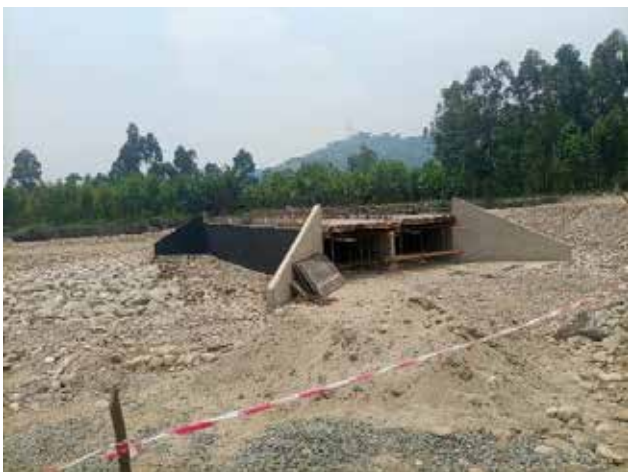
Kasese District: One of the box culverts under construction on the Karujumba Bridge
