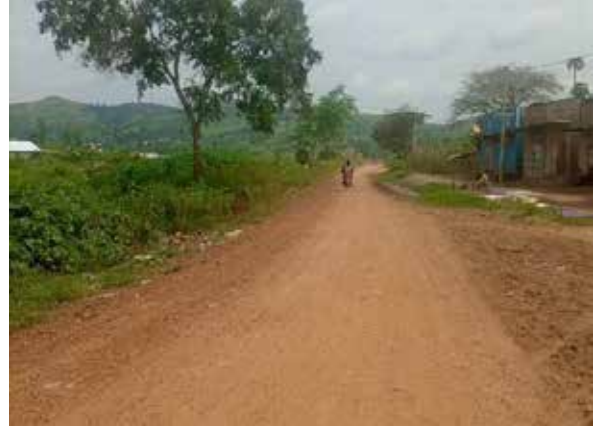
Lwengo District: A section of Kakyafu - Rwenkuma-Kyampalagata Road (8.5km) that was graded
