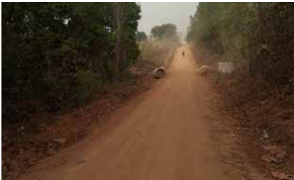
Hoima City: A section of Hoima-Kihukya Road at 8.2km was under periodic maintenance. Culverts were awaiting installation
