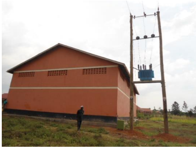
Installed 100 kva transformer in Butaleja District
