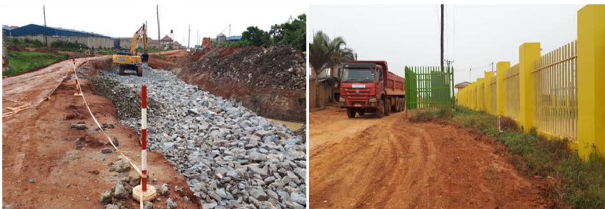
L-R: Ongoing civil works (rock filling), UMEME transformer erected in the road corridor at KIBP-Namanve
