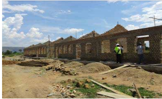
Ongoing civil works on three in one classroom blocks at Mbegu Primary School, Kikuube District
