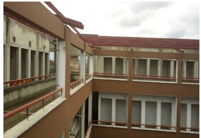
Incomplete roof covering in Mbarara Main Market
