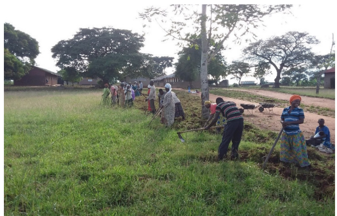
NUSAF3 labour intensive public works beneficiaries at work at Suni Primary School in Budaka District
