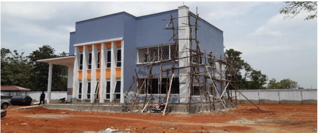
Left: Exterior works on Support to Teso Regional Office in Soroti District
