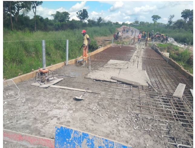
Casting concrete on bridge along Akara Hill-River Aswa-Cuku Community Access Road, Nwoya District
