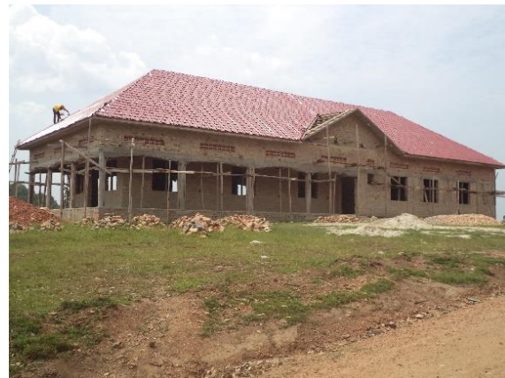
Incomplete super structure of new administrative building at Kyamuhunga sub-county, Bushenyi District as at February 2019
