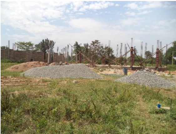
Raising of columns on new administrative block in Bulambuli District as at January 2019
