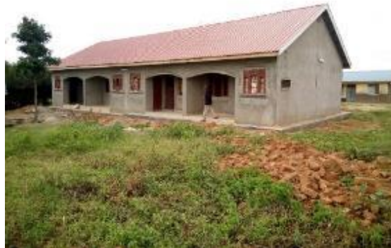
Incomplete four unit staff house at Kamaturu Primary School in Lorengedwat Sub County, Nakapiripirit District as at January 2019
