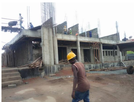
Steel work to columns on first floor for lockups ongoing as well as electro-mechanical works in progress, Kasese main market as at January 2019
