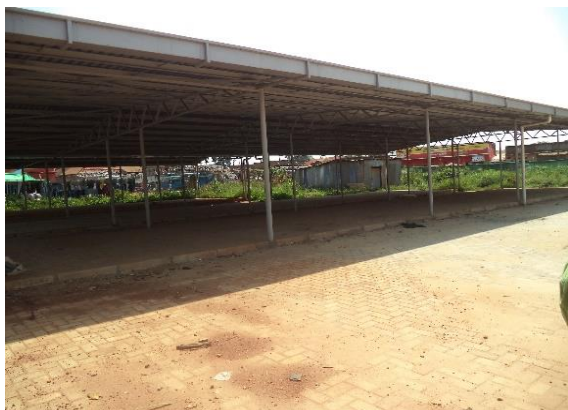
Incomplete paving works on parking area at the Nyendo market as at February 2019
