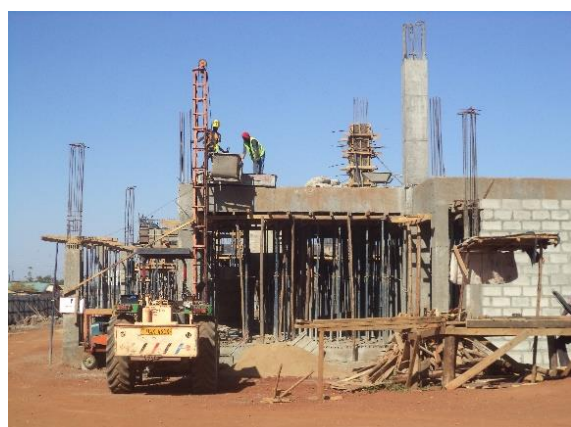
Ongoing construction works: Raising columns to roofing level at Loperu main market, Moroto Municipal at at January 2019
