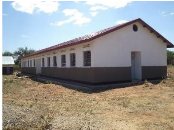
Completed Girls Dormitory in Karita Primary School, Amudat district as at January 2019
