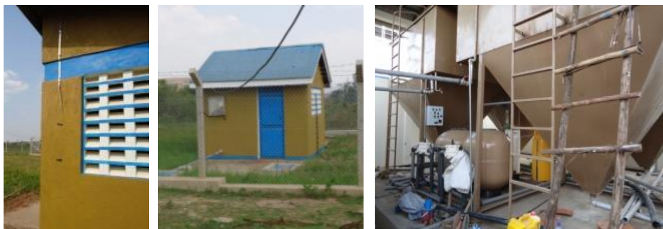
Left: Vandalized lightning conductor at Ginnery pump station; Centre: Renovated pump house at Abukol spring; Right: Dayliff treatment plant on Kachumbala mission hill
