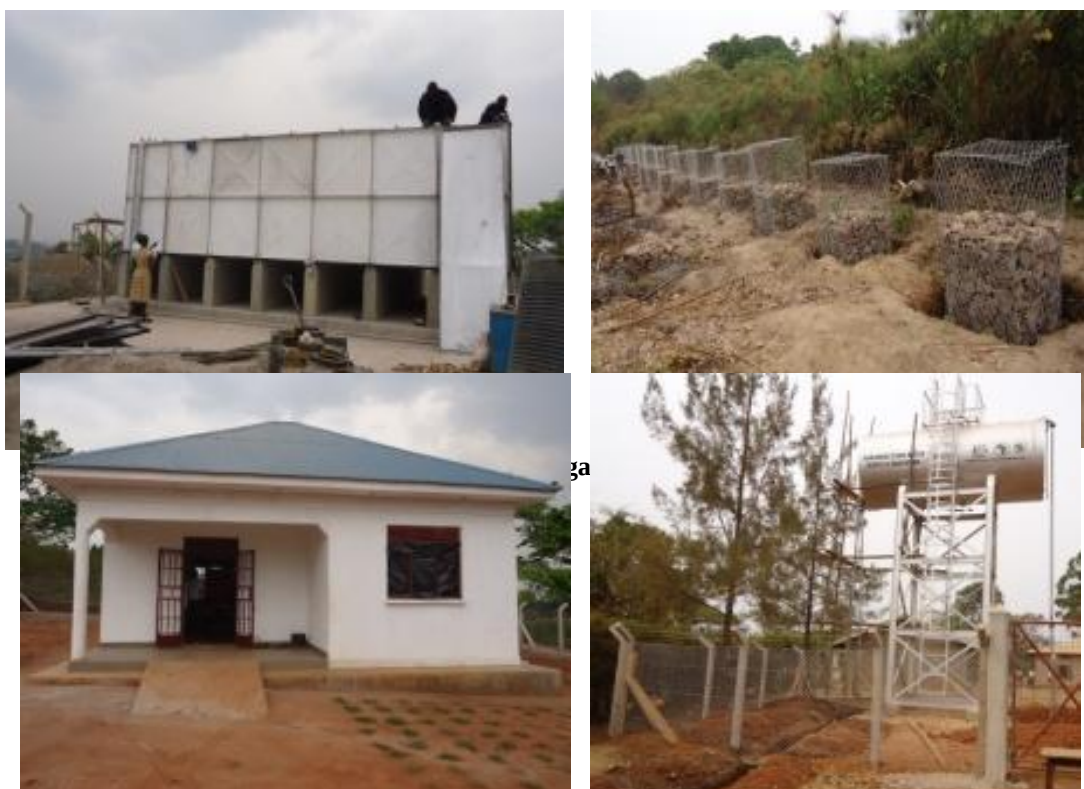
R-L: Water office in Kakumiro town council; 20m 3 reservoir tank at Kanyawawa Primary School
