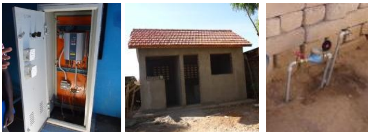
Left: Solar control at the pump station in Matany town; Center: Chlorine house in Matany town; Left: Household private tap in Matany town
