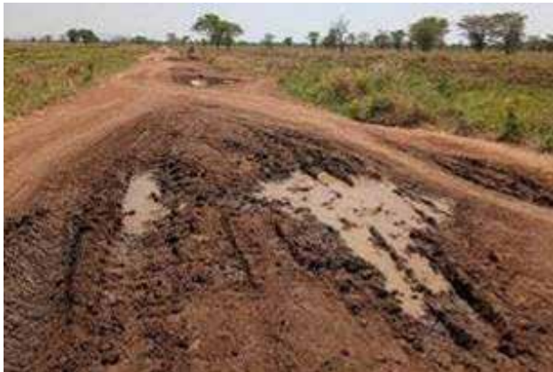
A defective ungravelled section along the Olekat-Matailong Road
