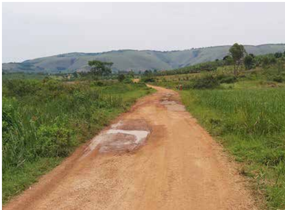
Swamp section along Nyakyera-Kibingo-Kitwe Road at Km 1+700 that had deteriorated due to heavy rains
