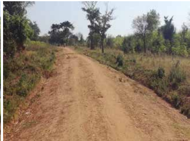
A well graded section of the Busembatita-Lumbuye Road just before the swamp works
