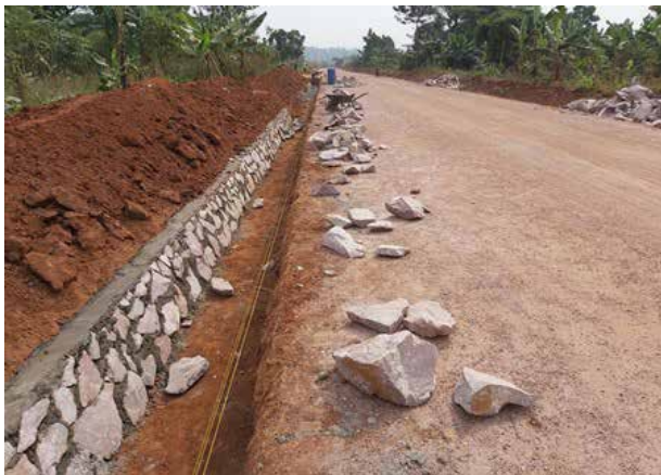
Stone pitching of side drains were ongoing along a primed section of Kasozi-Kifampa Road, Section A
