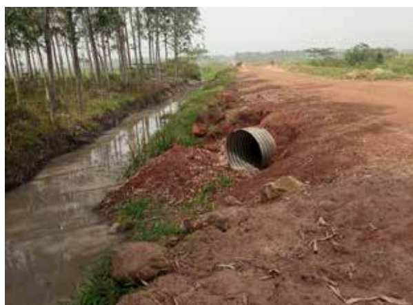
A swampy section of Mulanda-Nagongera Road at 5+400 with an installed armco culvert of diameter 1200mm
