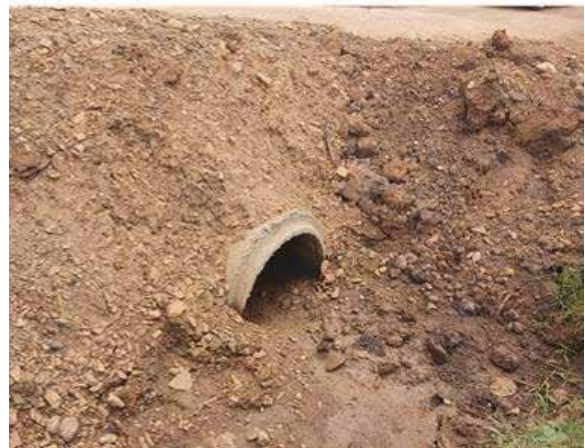
Sabya-Kitazigolokwa-Kinuuka Road: One of the installed culverts without end structures
