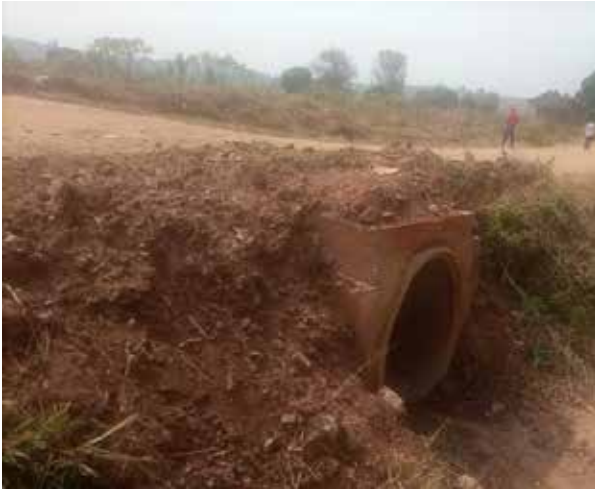
A section of Ocoke-Inde Road with an encased culvert installed at km 2+900
