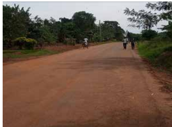
A sealed section at km 5+200 with edge breaking beginning to fanifest on the LHS of the road
