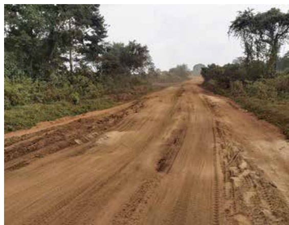
A section of Kayabwe-Bukasa-Muyanga Road at km 14+900 that had greatly deteriorated due to heavy traffic
