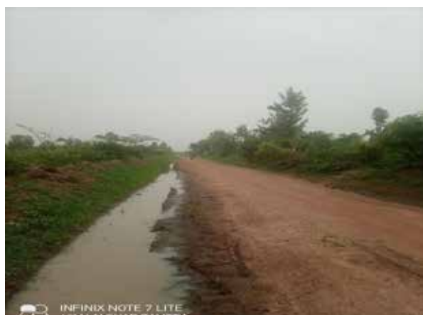
A section of Doho-Namulo Road at 0+000 showing effects of untimely drainage improvement that threatened to destroy the works.
