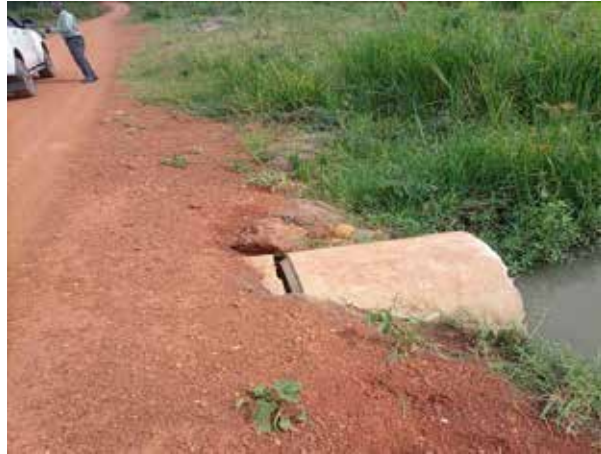
A raised section in the swamp Km 3+900 with culverts whose end structures were not yet constructed.
