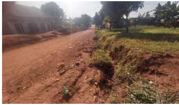
Part of the damaged side drain along Villa Maria–Kyamulibwa–Kabulasoke Road
