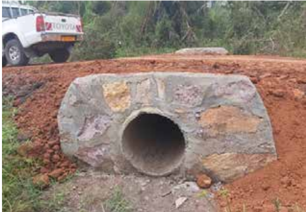
600mm diameter concrete culvert installed at the swamp section at Km 4+500 along the Nampuge-Bukasa-Kyonza Road
