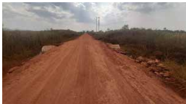
Incomplete installed culverts pending construction of headwalls along the graveled Masindi–Rwenkunya Road
