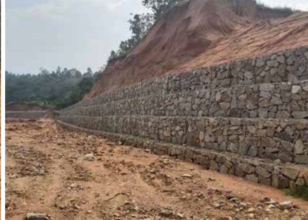
Gabion works installed to protect unstable slopes at km 35 along Rukungiri–Kihihi–Ishasha Road project
