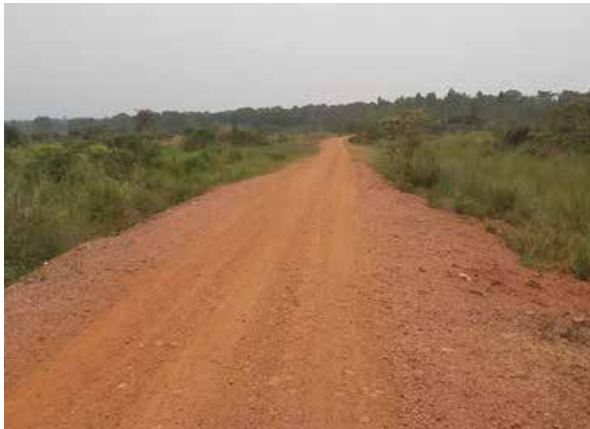
A swamp section from Ch 5+500 to Ch 5+560 on Kyampisi–Sombwe–Kyambogo Road(5.6km) was raised by 0.6m
