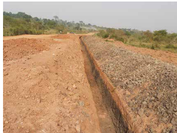
Excavation of a French drain in a swamp section along section B of Kasozi-Kifampa Road
