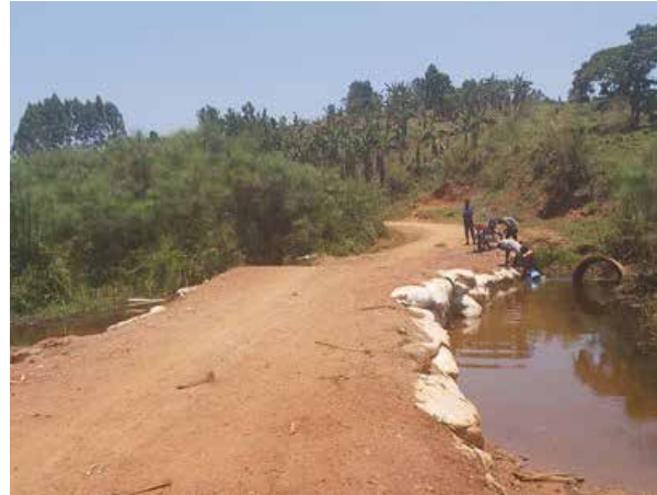
Ihunga-Kiryabyoma-Musambya-Bufungyo Road: Swamp raising and installation of 3 lines of culverts at Km 1+300
