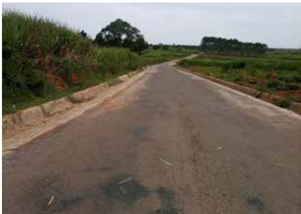
A sealed section of the road with stone pitching of side drains on both sides of the road at km 0+000
