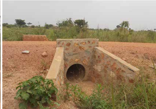
Double lines of 900mm diameter concrete culverts installed on Kibale - Kikamulo Road
