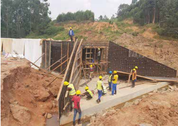
Construction of a box culvert on ) Rukungiri – Kihihi – Ishasha Road project at km 35+050
