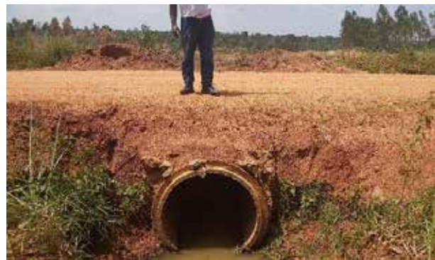
Incomplete culvert without headwalls along Kisuule–Nakaseke–Kapeeka Road
