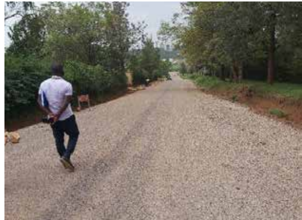
Kijjukizo Road after receiving the first seal of double bituminous surface dressing (DBST)
