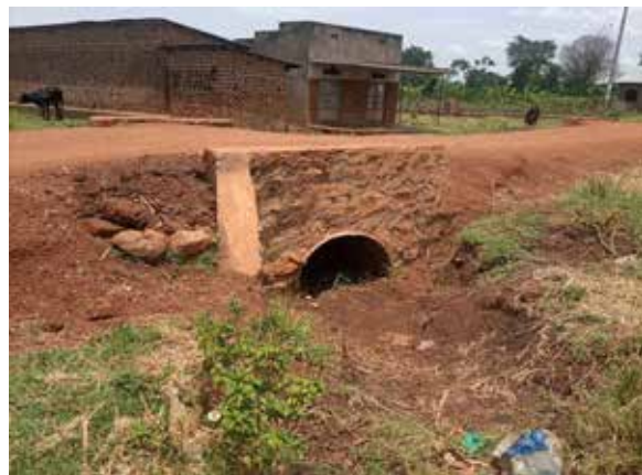
A silted culvert installed along Nakiwulo-Kitayundwa Road at Km 3+500.
