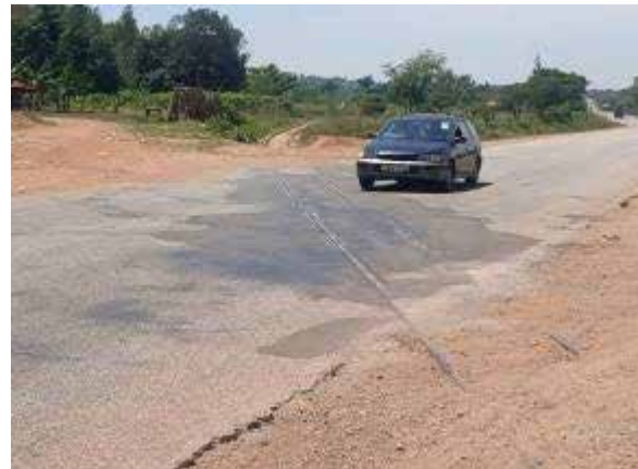
Pot hole patch works near a railway line at 4+300 on Tororo-Mbale-Soroti Road(150.8km) – Lot 1
