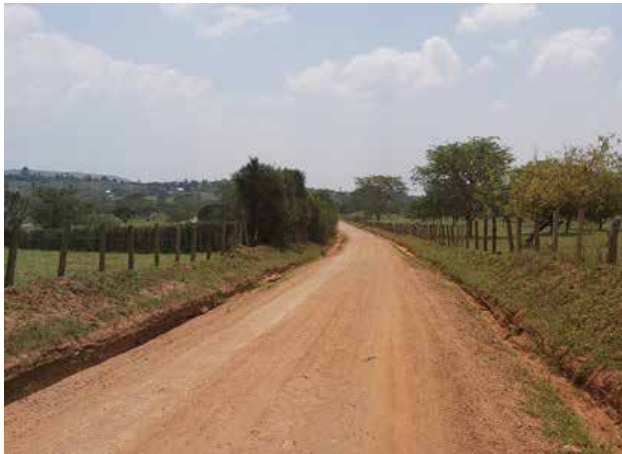
A gravelled section of Sabya-Kitazigolokwa-Kinuuka Road (18km) after emergency works in Q1
