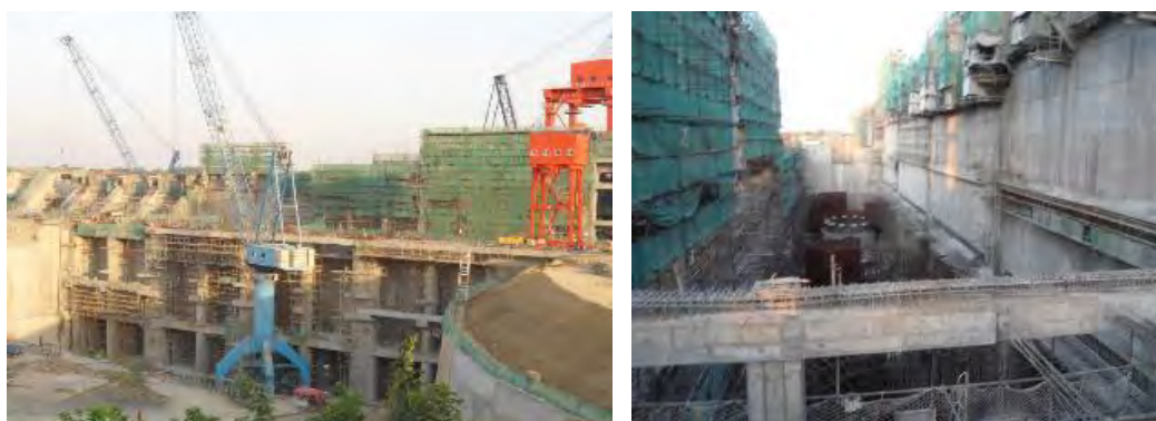
L: R: On-going civil works on the dam structure at Isimba HPP as seen from the tailrace; Civil works for the generator foundations in the powerhouse at Isimba HPP
