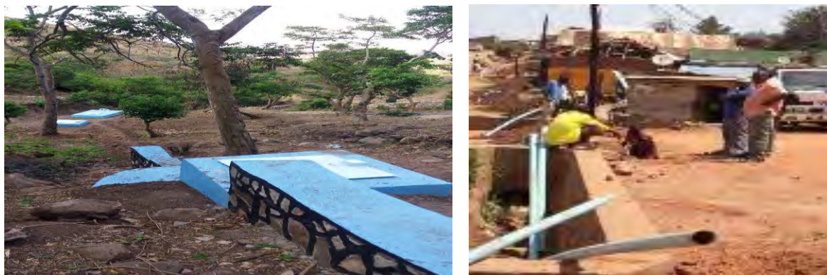
L-R: Protected water catchment at Murema water source; Community members excavating water trenches and laying pipes for the water source at Kashumba sub-county, in Isingiro district
