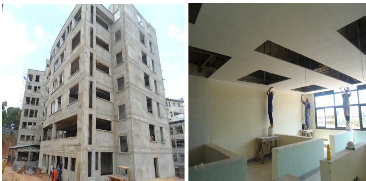
L-R: On-going construction works at the maternal and neonatal unit; Painting of the children's ward
