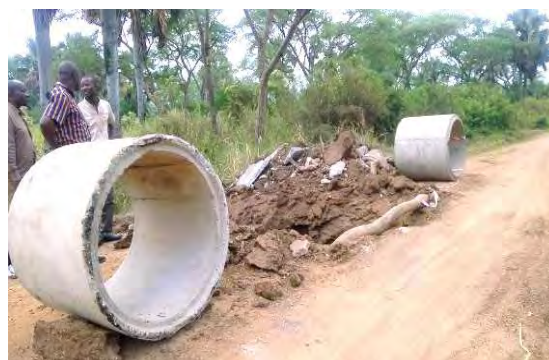
Culvert installation works ongoing along Karugutu – Ntoroko road spilled to quarter three
