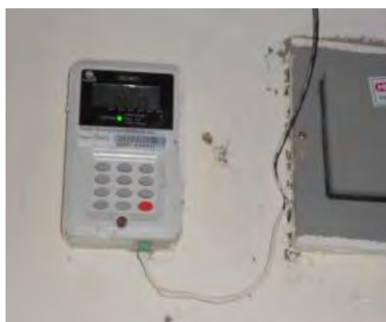
User interface unit on one of the OBA connections made by Kyegegwa Rural Electricity Cooperative Society in Kyegegwa district
