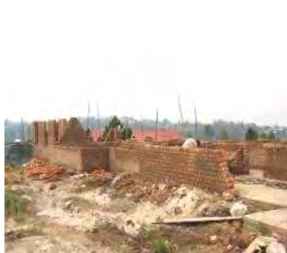
Ongoing construction of the Production Department Office Block at Kunywa Village, Mityana Municipality using PMG funds
