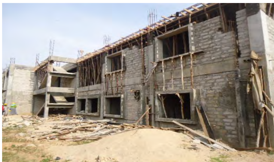
On-going construction works for the Paediatric and Maternity ward at Masaka RRH
