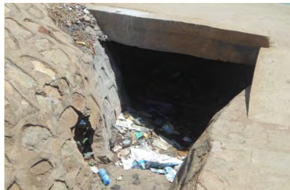
Blocked newly constructed drainage channel in Mbale town along Nakalama-Tirinyi-Mbale Road
