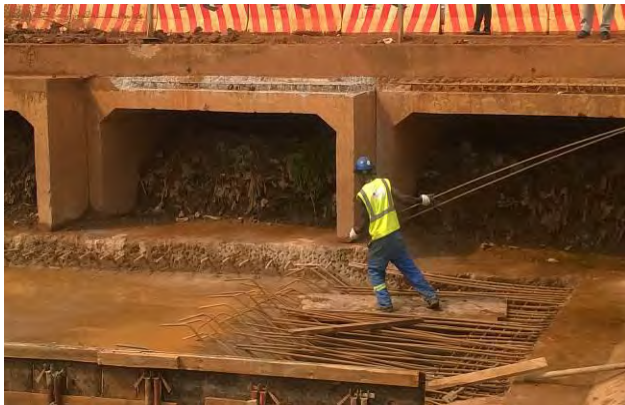
A newly constructed clogged box culvert supposed to discharge water into Lubigi channel, Northern Bypass
