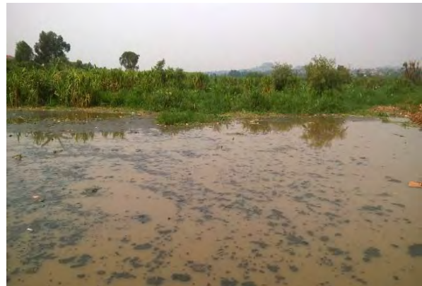
Stagnant water downstream the Lubigi Channel at the Hoima Road junction section
