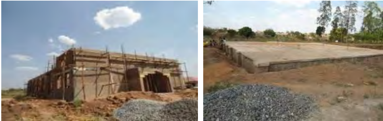
L-R: On-going civil works on the church; Foundation for the mosque at Karuma, in Kiryandongo/Nwoya district
