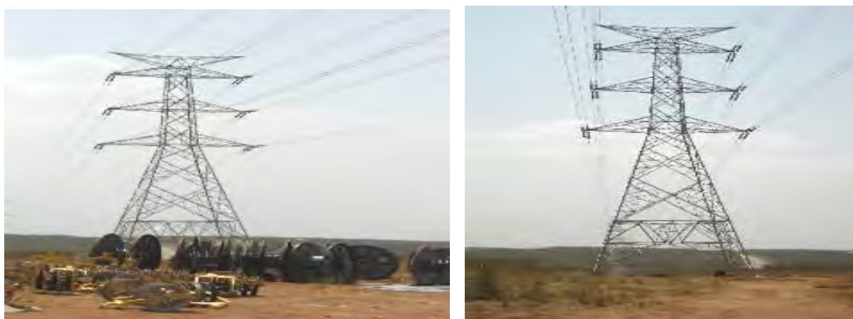
Recently strung section of the Hoima-Nkenda transmission line in Hoima District
