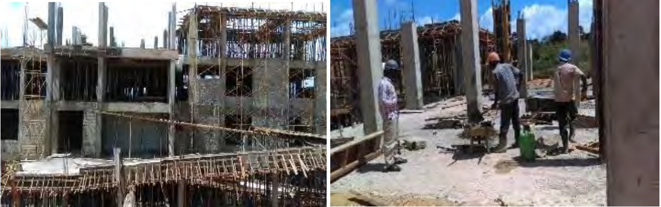
L-R: Construction works of new Engineering Workshop at ring beam level with structural works completed at 90% at Kyambogo University
