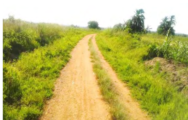
Bush covering part Bulingo-Kalangala landing site road due to lack of routine manual maintenance
