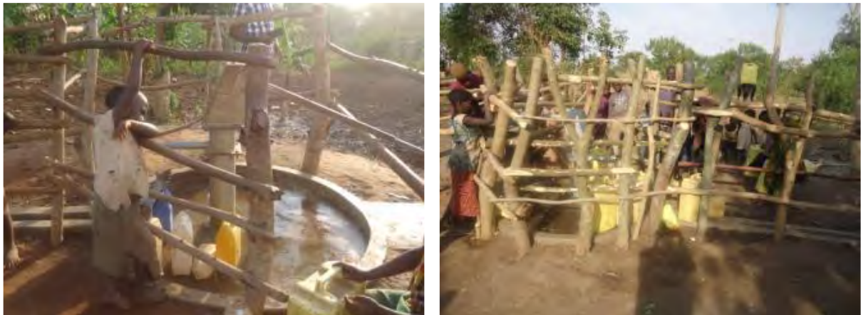
L-R: Newly constructed borehole: Kakonge borehole in Kakonge village Namingo sub-county; Nakibuya borehole in Kasodo sub -county
