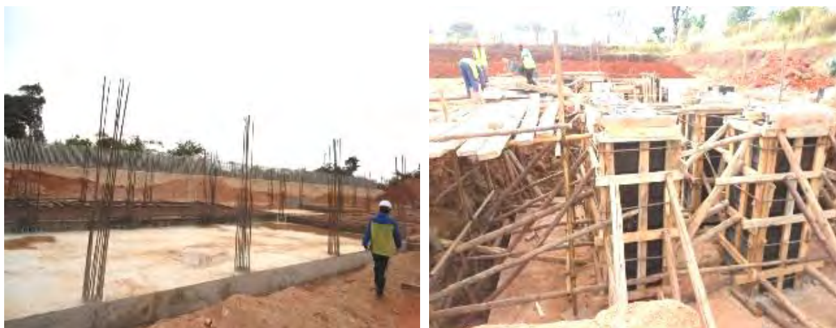
L-R: Foundation works for the plant house in Hoima substation; Civil works for equipment and overhead gantry foundations at Nkenda substation
