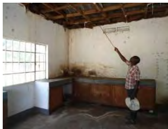
Dilapidated office and laboratory block under use at Nshaara Ranch in Nyakashita Parish, Kiruhura district. Staff were demotivated working from these structures
