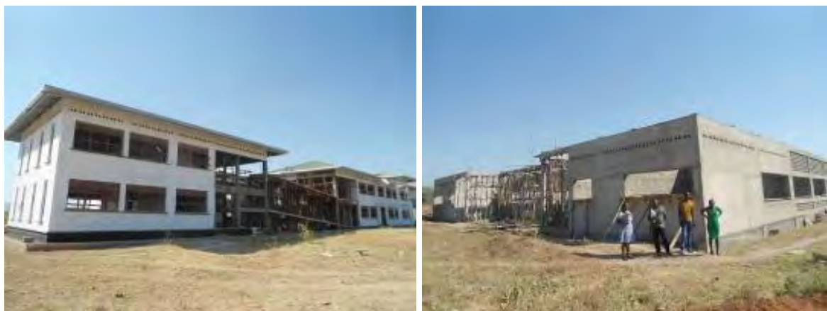
L-R: Some of the stalled structures at Amelo T/I in Adjumani. The main workshop block
