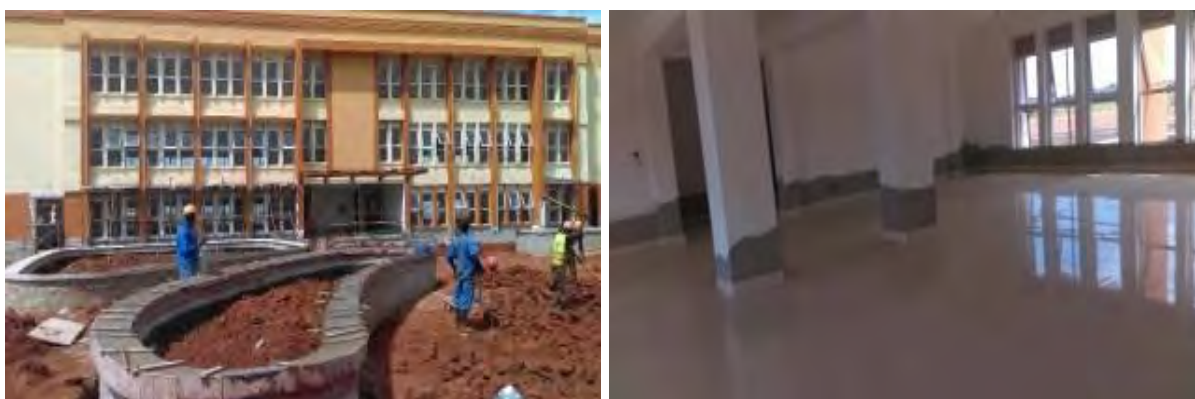
L-R: Outside view of Administration block; Section of the Library awaiting furnishing at Uganda Petroleum Institute Kigumba in Kiryandongo District
