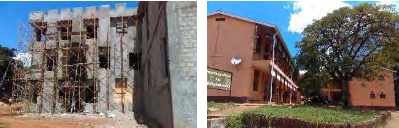
L-R: Multi-purpose science lab with structural works at 100; renovation works at the Department of Civil and Building Engineering complete and handed over at Kyambogo University
