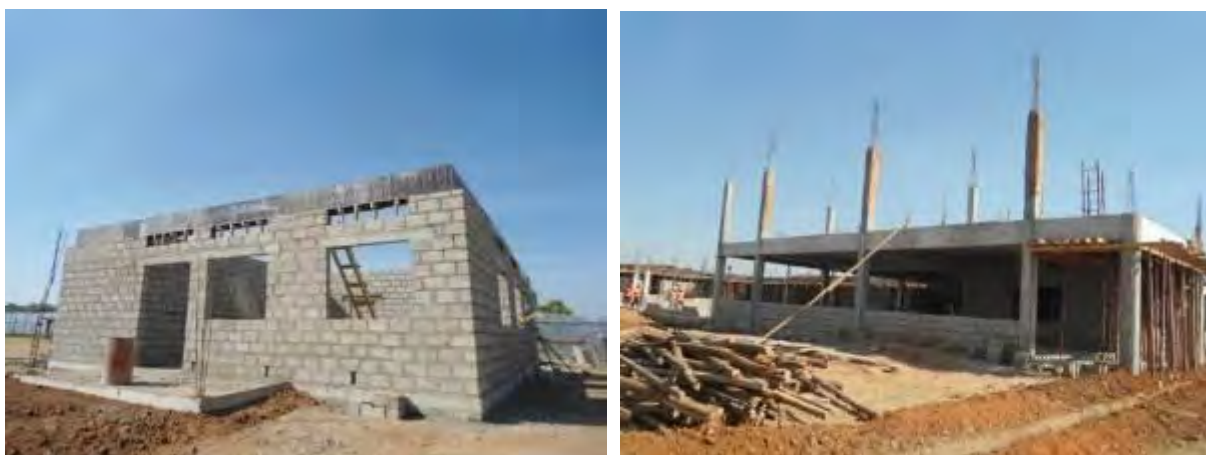
L-R: The Utility Block at 60% progress; and Science Block at 50% progress at Muni University
