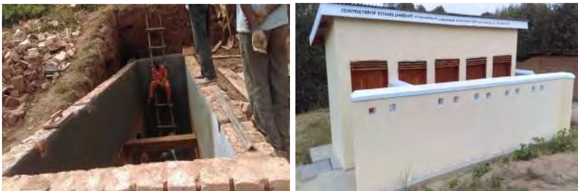
L-R: A 5-stance lined pit latrine under construction at Katuna P/S; Kabale District; Completed 5 stance lined pit latrine at Rwatabaire P/S; Ishongororo Subcounty; Ibanda District.
