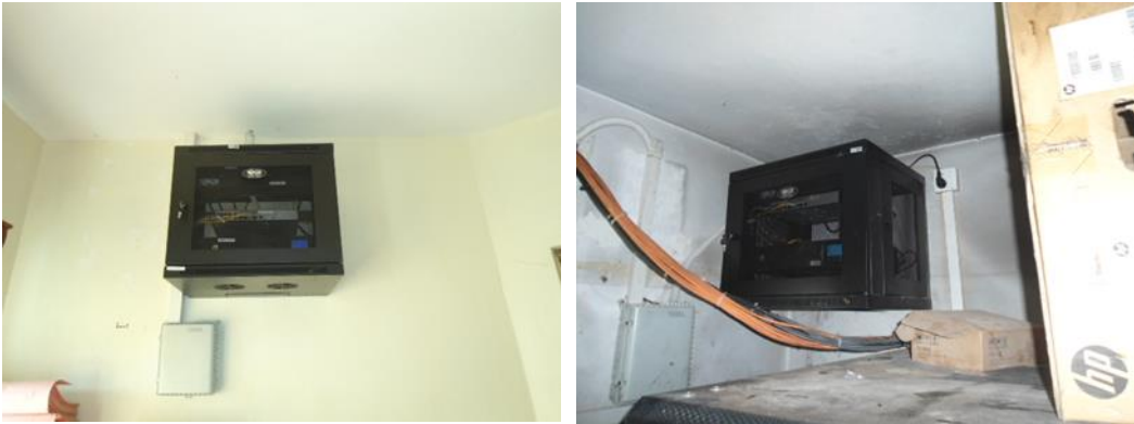
L-R: Routers installed at Kumi Judicial Offices and Marie Stopes- Tororo under the Last Mile Connectivity of the RCIP that are not utilising services over the NBI as at 28 th May 2021
