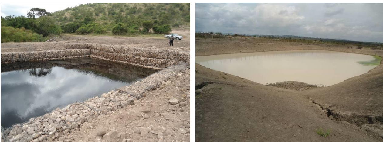
The water reservoir (left) and one of the valley dams that were constructed by the MAAIF project at the NEC farm in Kisozi Village, Gomba District
