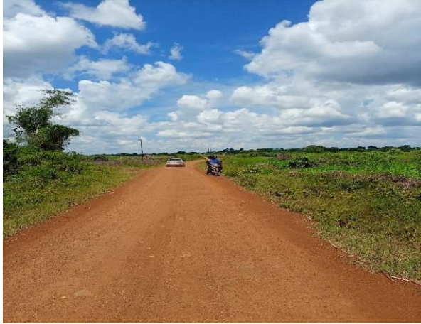
A section of Ngandho-Buyamba-Iraapa Road at Km 0+500 in Buyende District that was well graded and graveled
