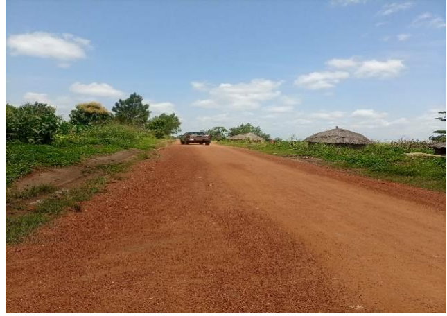
A well-shaped and graded section of Korom-Pece-Labora Road at km 0+000 at Labora off Gulu-Moroto road in Gulu District
