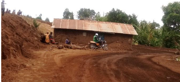
A project affected person (PAP) awaiting compensation at 41+000 on Kapchorwa-Suam Road; causing delay in site possession
