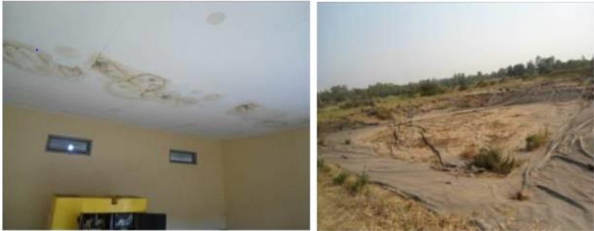
Shoddy works of leaking roof of the power house (left) and dilapidated polythenes in the water ponds at Gulu Aquaculture Centre in Laliya Village, Loro Division in Gulu District
