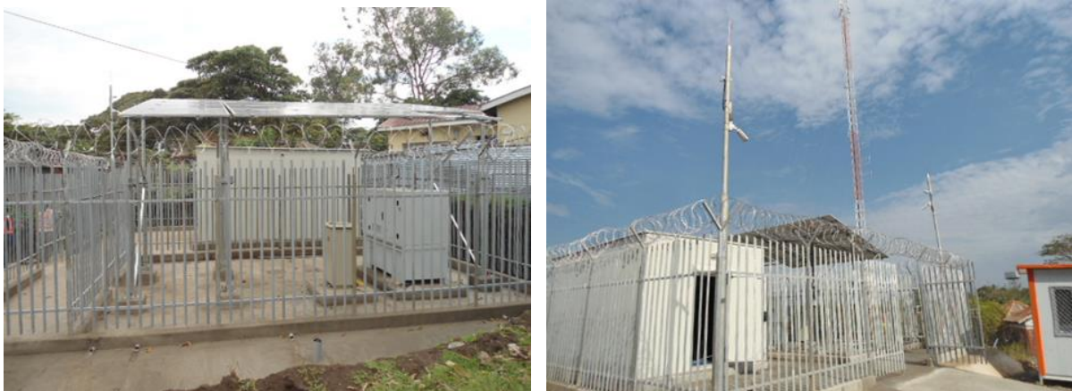
Transmission sites at Mpondwe border and Koboko constructed under the Missing Links Project
