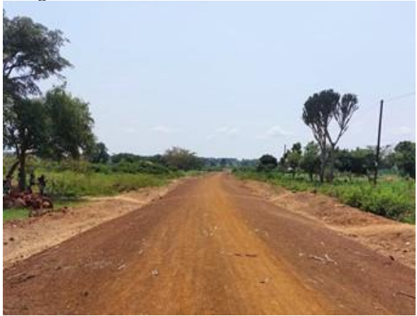
A section of Kisarisi-Kiwenda (2km) was well graded and graveled in Kayunga District
