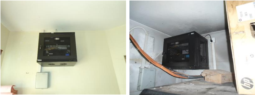
L-R: Routers installed at Kumi Judicial Offices and Marie Stopes- Tororo under the Last Mile Connectivity of the RCIP that are not utilising services over the NBI as at 28 th May 2021
