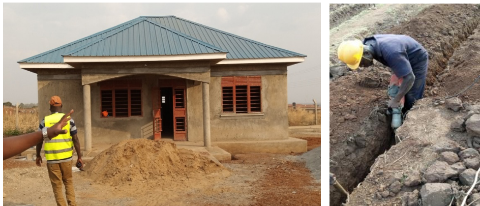
L-R: A twin tank of 200m 3 concrete and a water borne toilet with an incinerator at a market in Kiyindi, Kihindi Town Council, Buikwe District
