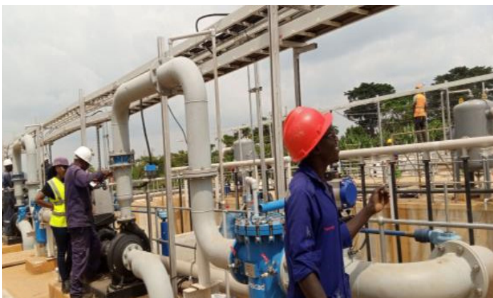
L-R: Electro Mechanical works ongoing at the Water Treatment Plant in Katosi
