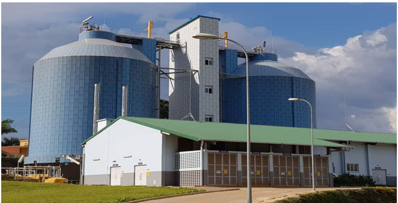
The two bio digesters (blue) and in front is the power generation house
