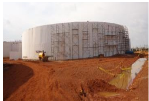
One of the four 10,000m 3 Reservoir Tanks at Nsumba Hill in Mukono District
