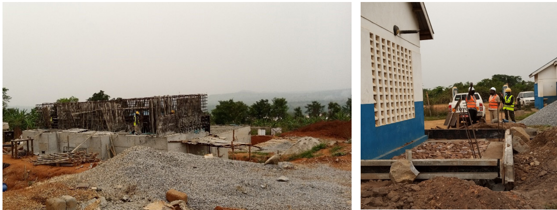
Ongoing works at the treatment plant and source expansion in Kapeeka WSS, Kapeeka Sub-county Nakaseke District
